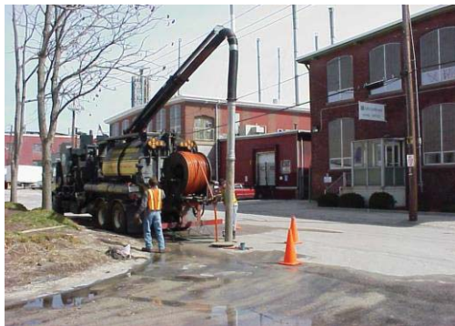
Photo: Interceptor Grit Removal
