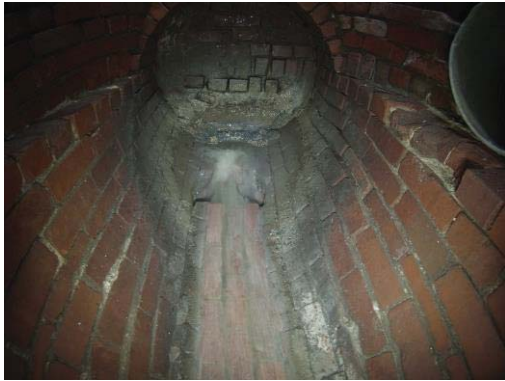
Photo: OF 056 Regulator on Vandewater Street
