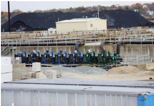
Photo: Aeration Tank Pumps
