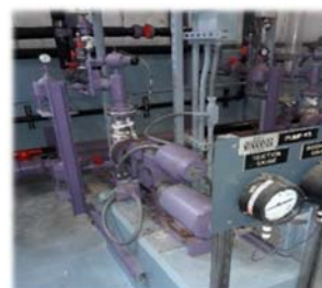
Photo: Bisulfite Pump at Field's Point
