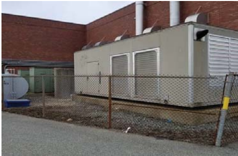
Photo: Field's Point Screw & Blower Generator
