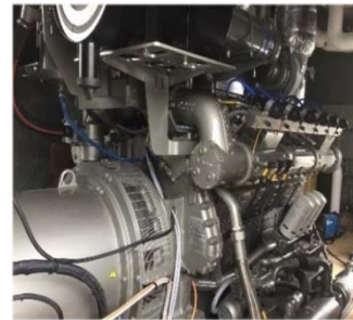
Photo: Bucklin Point Biogas Facility
