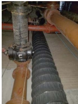
Photo: Digester #2 Vent Hose #4
