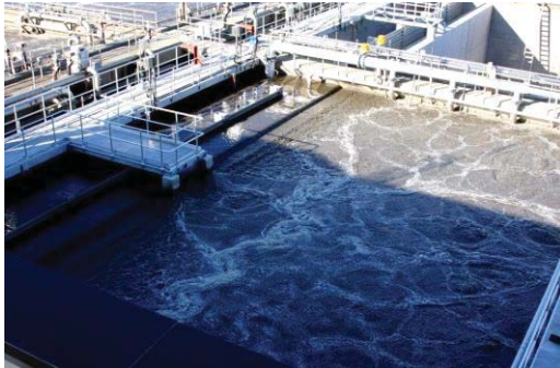
Photo: Aeration Tanks at Field's Point WWTF
