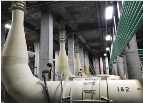
Photo: Inside Ernest St. Tunnel Pump Station
