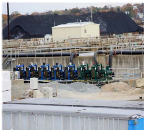
Photo: Aeration tank pumps at Field's Point
