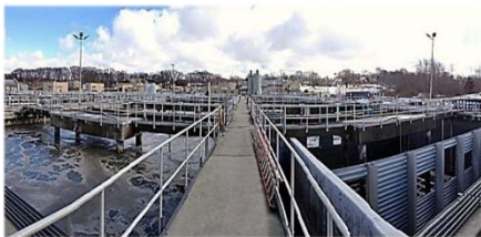
Photo: Aeration Tanks at the Field's Point Wastewater Treatment Facility
