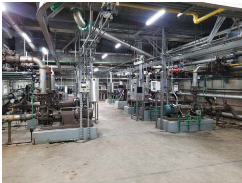
Photo: Primary Pump Station
