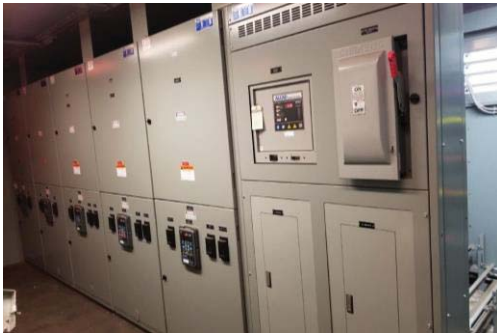
Photo: Field's Point Electrical Facility
