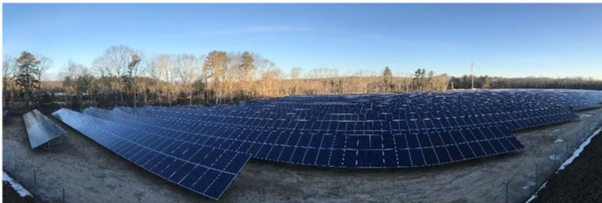
Photo: NBC's Solar Facilities in North Kingstown, RI
