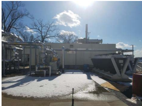
Photo: Bucklin Point Biogas System
