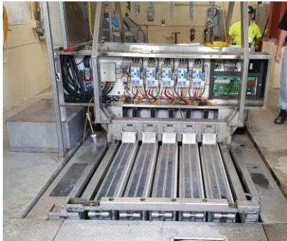
Photo: Bucklin Point UV Disinfection System
