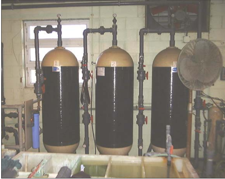
Copper Recycle Ion Exchange pretreatment system at Tri-Jay Jewelry Company
