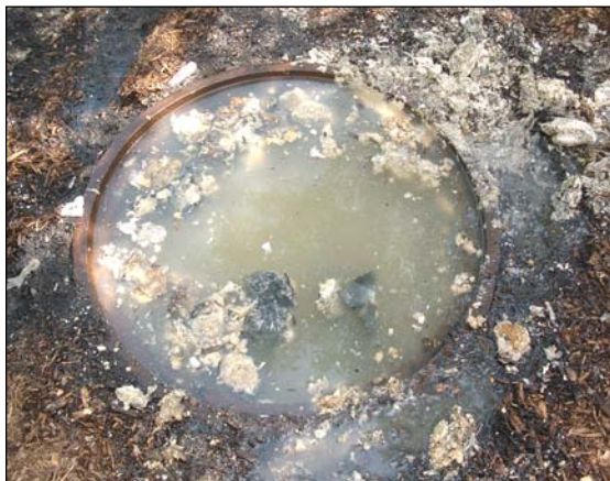
Blockage due to poor maintenance on Passive Grease Traps
