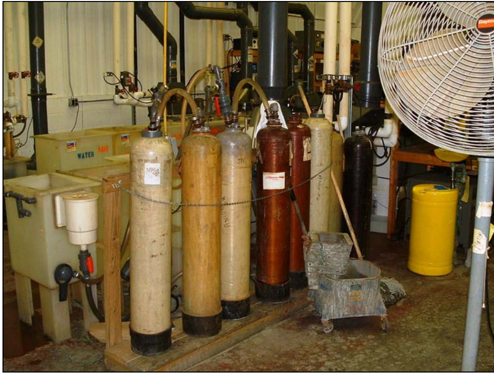
Part of an Ion Exchange System at a Permitted Zero Discharge Facility
