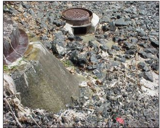
Surcharging manhole due to a grease and solids blockage
