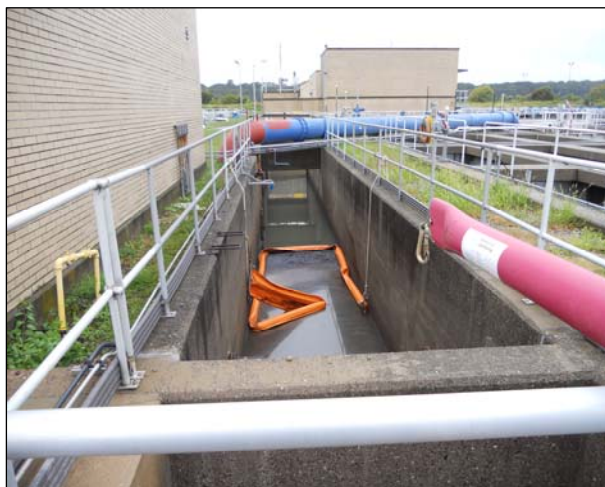
Boom Deployed in the Chlorine Contact Tank
