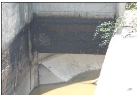
Wet Weather Influent Channel Gate
