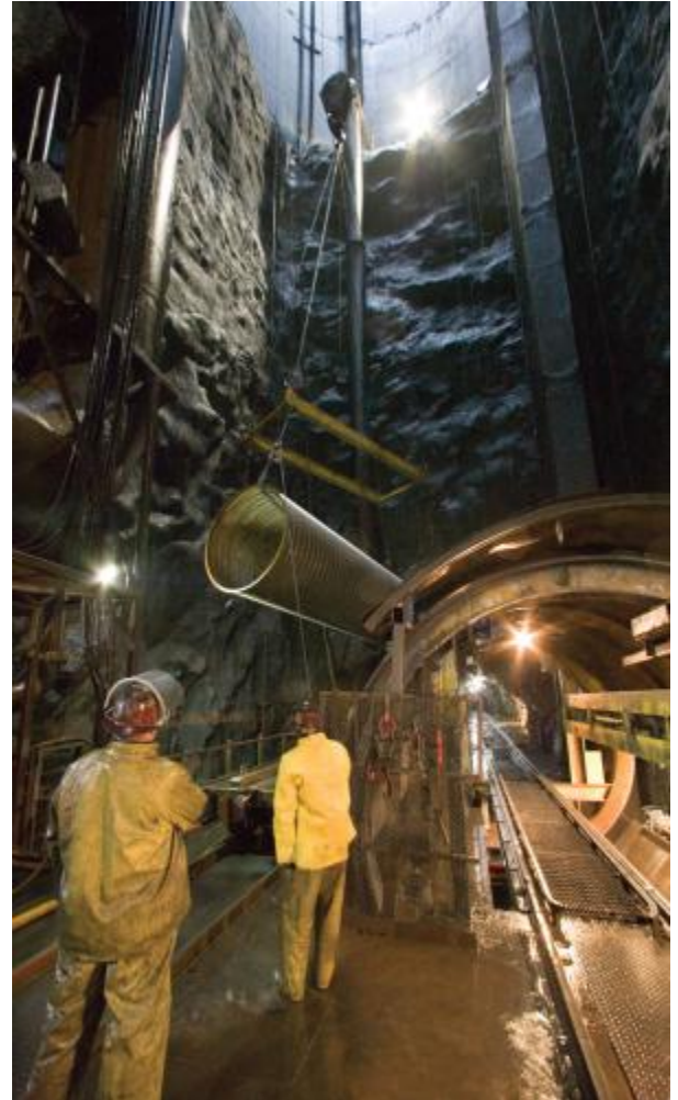
Workers lower ventilation components into the Deep Rock Tunnel during construction. As the tunnel boring progressed, necessary utilities such as electricity and fresh air also had to be built forward.
