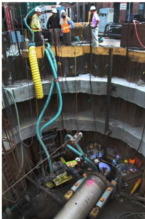
The large multi-story hole at Kinsley Avenue and Eagle Street in Providence, where 36-inch pipes are being connected as part of Phase II of the Combined Sewer Outflow Project.
