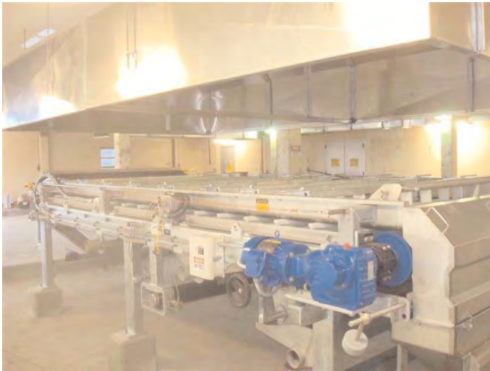
New Gravity Thickener at Bucklin Point.
