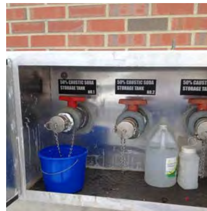
Field's Point Caustic Soda Tank Fill Valves
