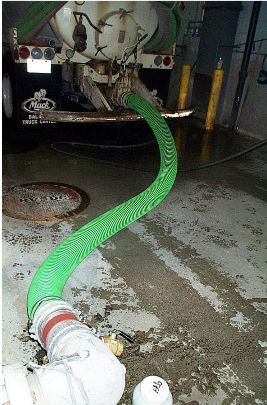
Septage sampling valve installed on discharge coupling
