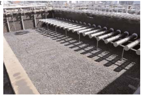
Millions of plastic media covering the bottom of the empty IFAS tank.
