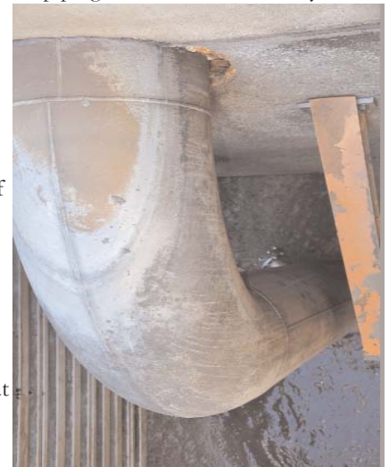
Pipe where the air-leak was coming from.
