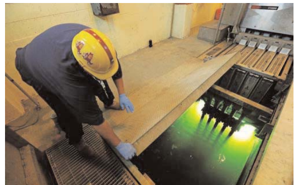
Ed Taylor inspects the UV disinfection system
