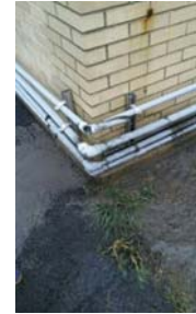
Broken RAS Line
