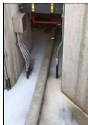
Fire Foam Secondary Containment
