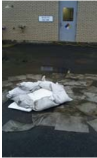
Protected Catch Basin
