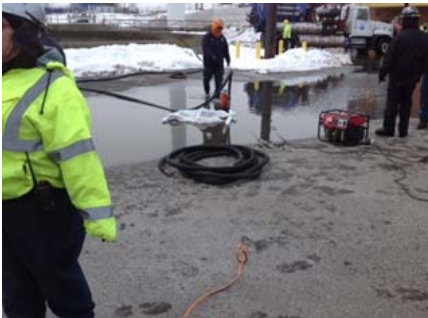
Primary Sludge Spill at Field's Point
