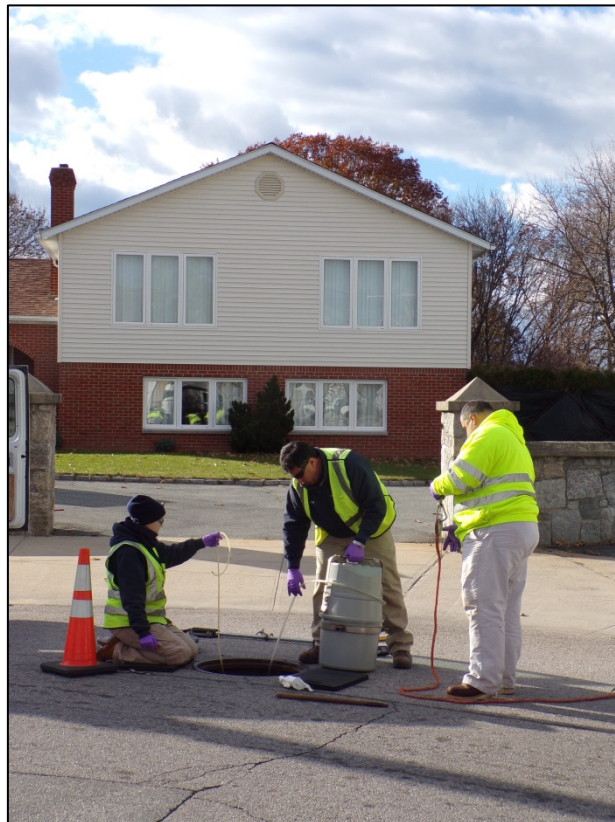
Sanitary Manhole Sampling
