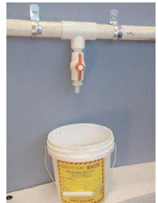
2. Always flush valve briefly and safely before sampling
