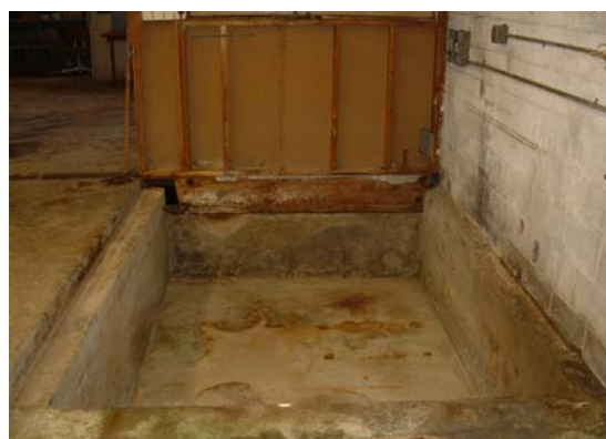
Follow-up inspection of the same facility to verify that the firm has disposed of all solutions and complied with NBC Shutdown Procedures.
