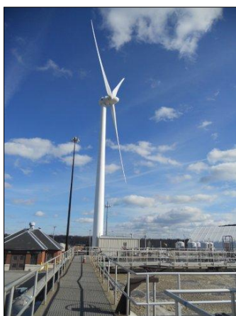
Field's Point Wind Turbine and IFAS Tank
