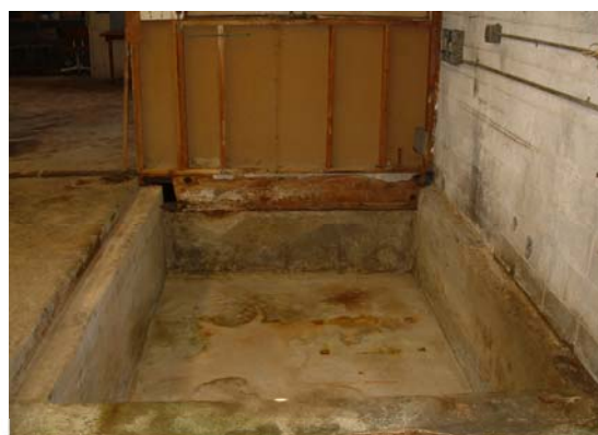
Follow-up inspection of the same facility to verify that the firm has disposed of all solutions and complied with NBC Shutdown Procedures.
