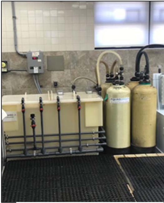
Part of an Ion Exchange System at a Permitted Zero Discharge Facility
