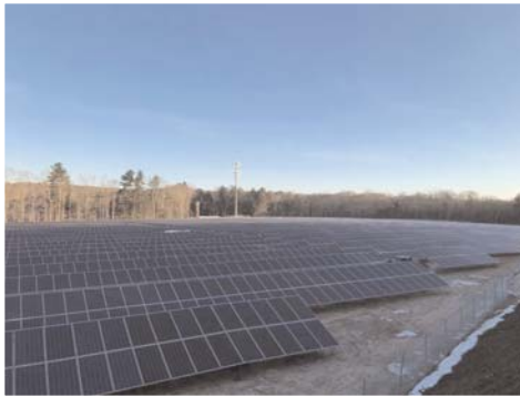
NBC Solar Array.
