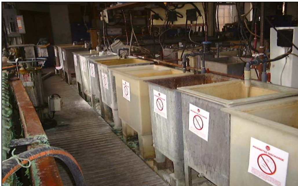
Tanks at a shutdown plating shop are stickered "PROHIBITED DISCHARGE"
