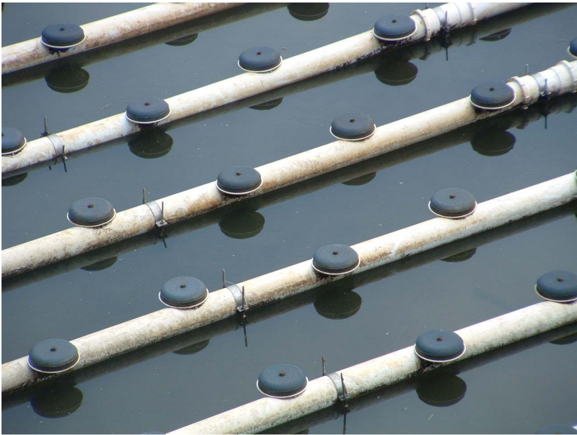
Photo: Field's Point Wastewater Treatment Facility aeration tank
