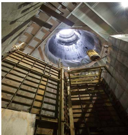
Photo: A view from the pump station cavern utility shaft looking up through stairway forms and a steel roof deck. The pump station floor is approximately 300 feet below the ground surface, the equivalent of a 25 story building.
