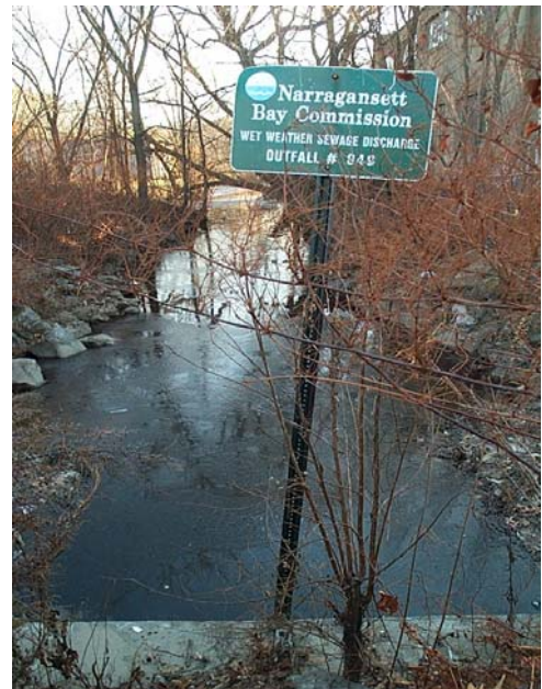
Photo: This combined sewer overflow is located in the Woonasquatucket River near Valley Street in Providence, and will be addressed as part of the Phase II facilities.
