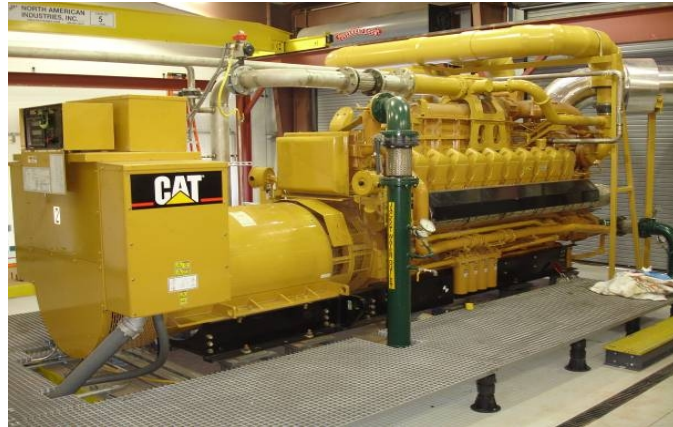
Photo: A Caterpillar reciprocating engine
