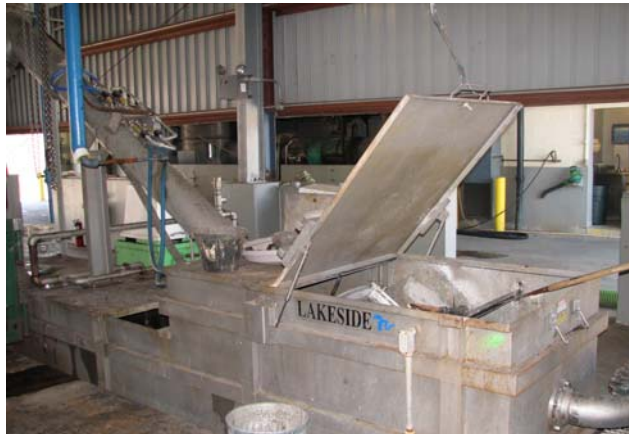
Photo: Lakeside Grit Removal Unit
