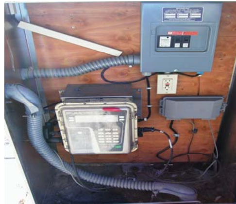
Photo: The Smith Street Permanent Meter Enclosure
