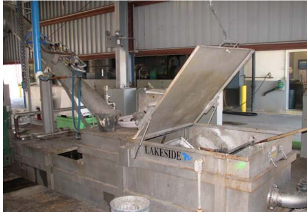
Photo: Lakeside Grit Removal Unit
