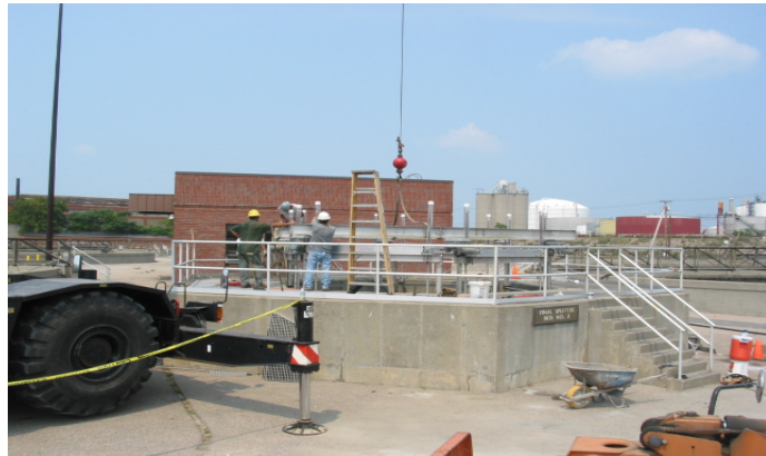
Photo: Replacing of final clarifier splitter box gates, built in the 1980's
