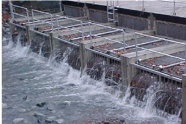
Photo: Floatables Control Facilities at Bucklin Brook
