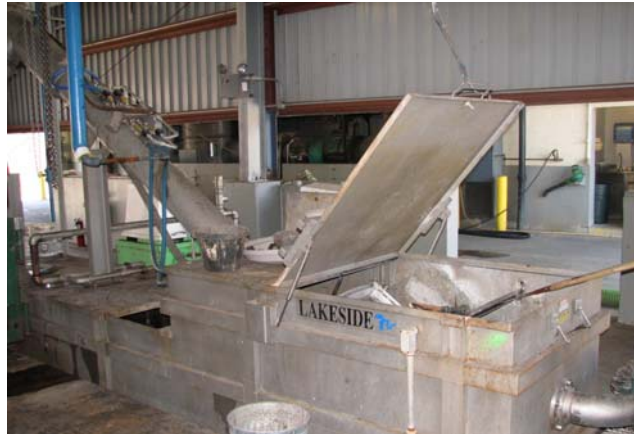
Photo: Lakeside Grit Removal Unit
