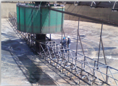
Photo: Inspection of a Field's Point Clarifier to be upgraded as part of the nitrogen removal project
