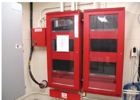
Photo: An existing fire alarm panel from one of NBC's buildings
