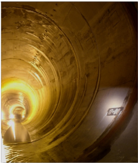
Photo: A view of a portion of the completed three mile long CSO Tunnel
