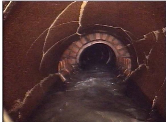
Photo: Clay Interceptor in need of replacement
