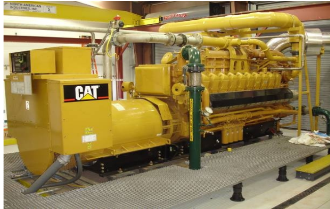
Photo: A Caterpillar reciprocating engine
