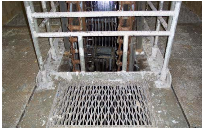
Photo: Bar screen in the Omega rack room
