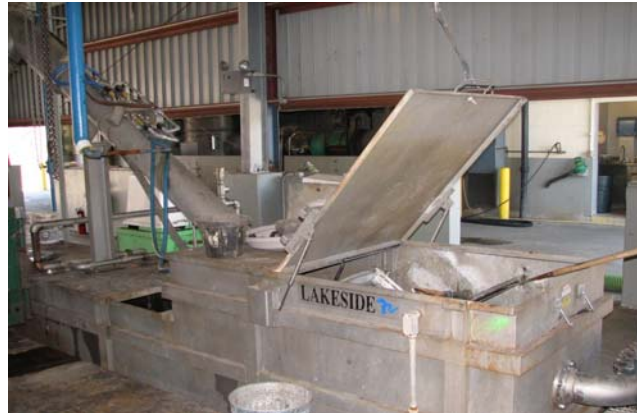
Photo: Lakeside Grit Removal Unit
