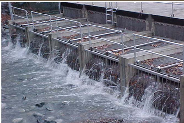
Photo: Floatables Control Facilities at Bucklin Brook
