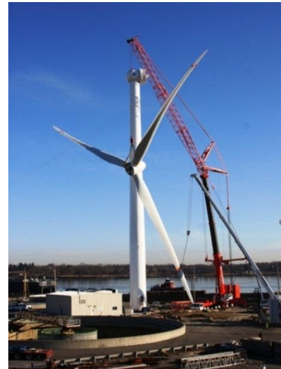
Photo: Field’s Point wind turbine
