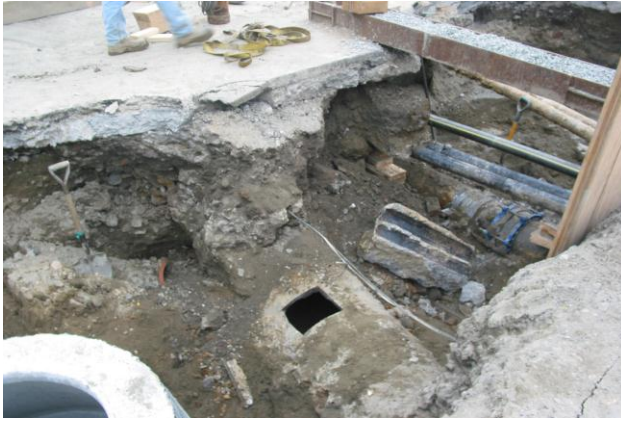
Photo: Removal of abandoned pipe at Atwells Ave. and Valley Street Project Overview
