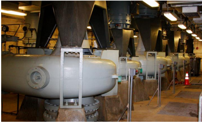
Photo: Motors at the Ernest Street Pump Station Project Overview
