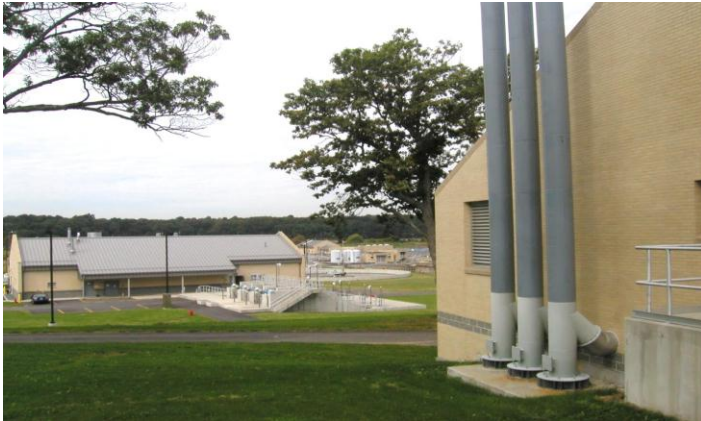
Photo: Bucklin Point Boiler Stacks
