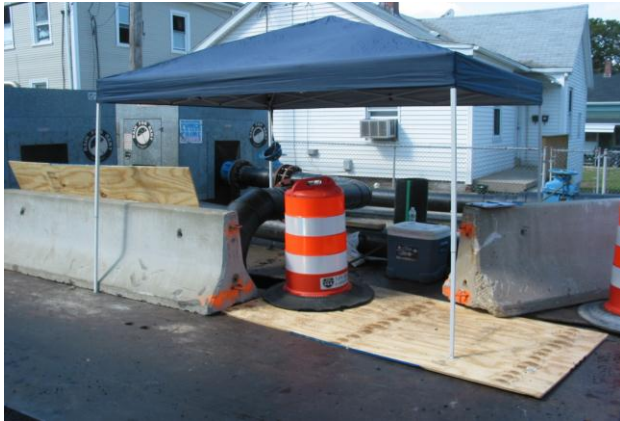
Photo: The intake and discharge piping on Branch Avenue Project Overview
