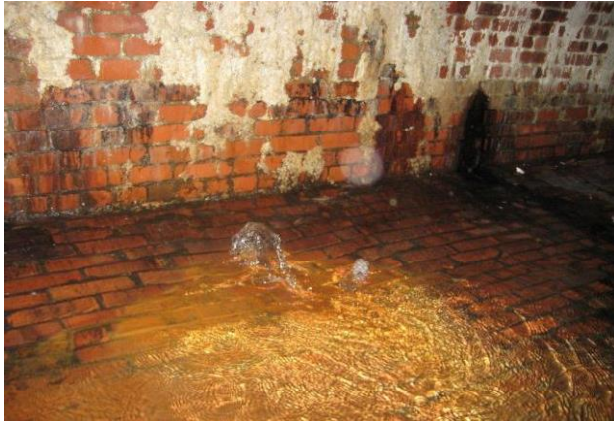
Photo: Infiltration into existing WC3O3North overflow Project Overview
