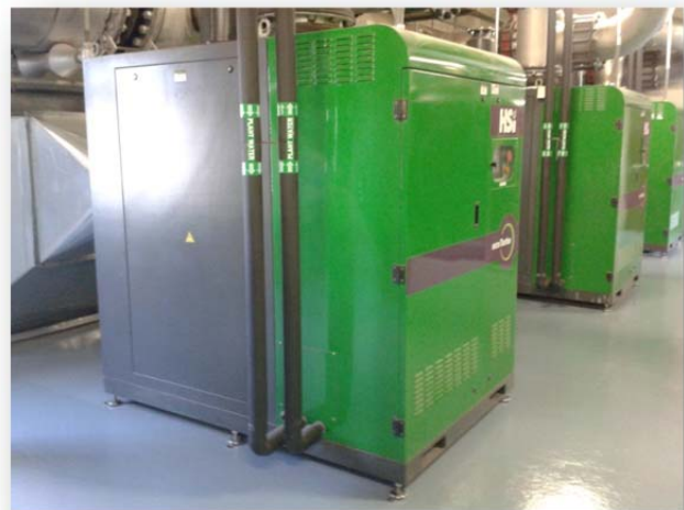
Photo: New turbo blowers at Field's Point
