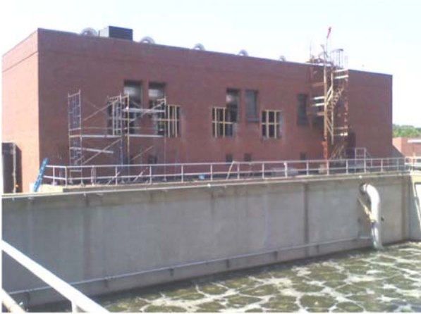
Photo: Blower Building Louver Cut-outs
