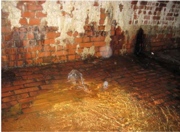
Photo: Infiltration into existing WCSOI North overflow
