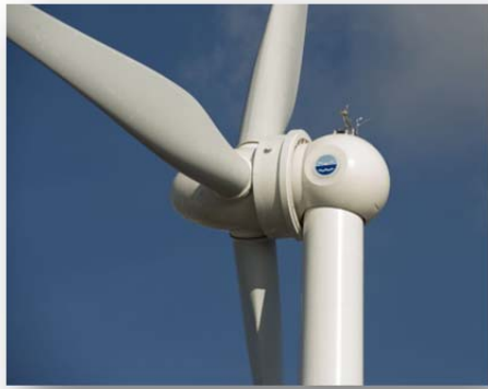
Photo: FPWWTF Wind Turbine
