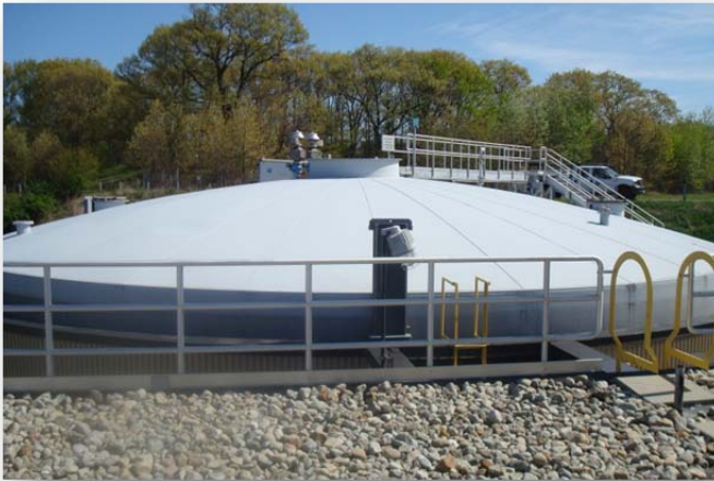
Photo: Digester tank at Bucklin Point
