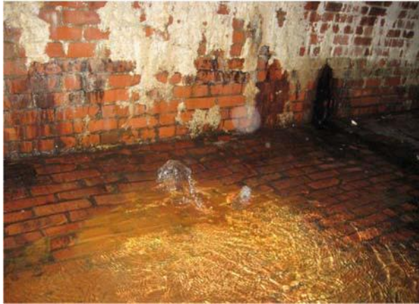
Photo: Infiltration into existing Woonsocket North overflow
