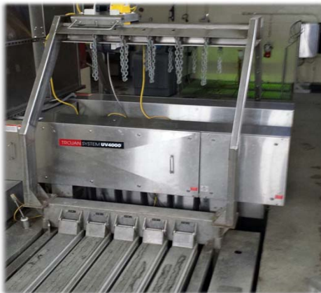
Photo: UV System at BPWWTF
