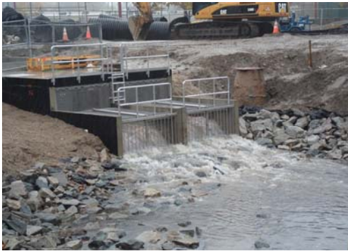
Photo: Trash Net Facility at OF 220
