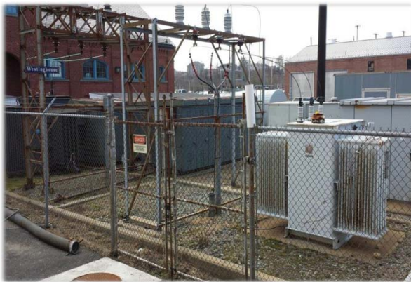
Photo: Field's Point Main Electrical Substation
