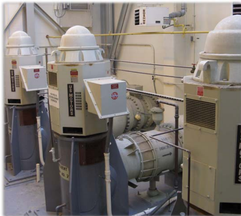
Photo: BPWWTF Effluent Pumps
