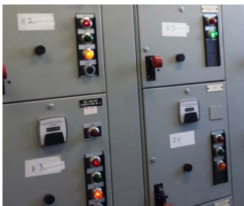
Photo: Electric Panel at FPWWTF
