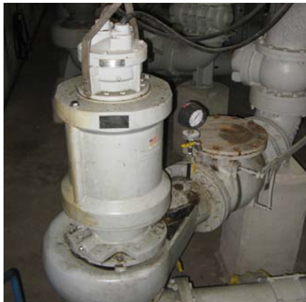
Photo: Pump at Omega Pump Station
