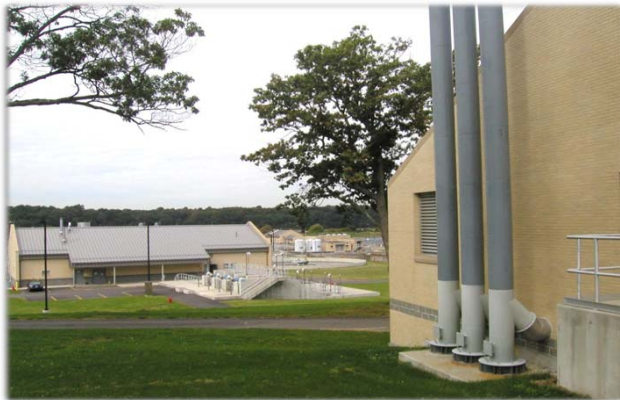
Photo: Bucklin Point Boiler Stacks
