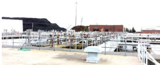
Photo: FP Blower Building
