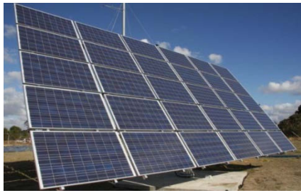
Photo: Solar Photovoltaic Energy Array
