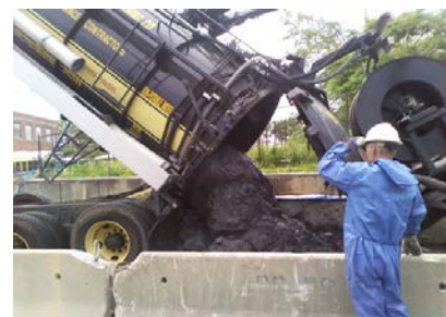
Photo: Interceptor Grit Removal
