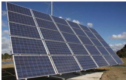
Photo: Solar Photovoltaic Energy Array
