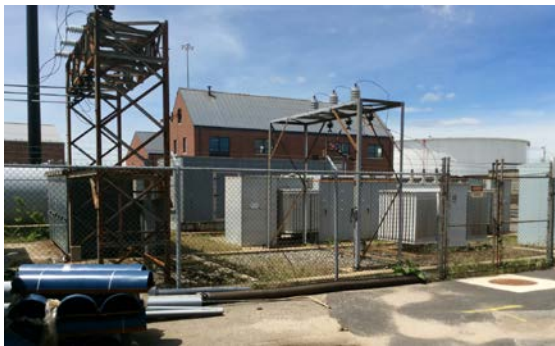
Photo: Field's Point WWTF Electrical Substation #1
