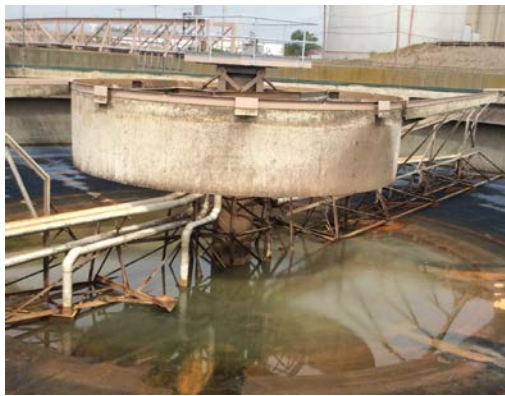
Photo: Final Clarifier at FPWWTF
