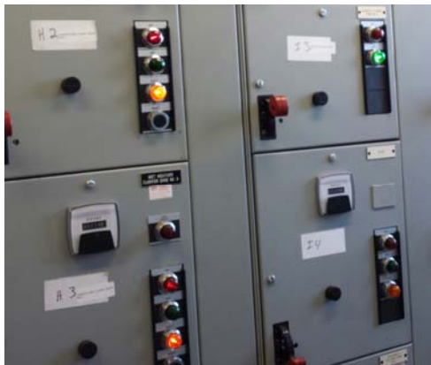
Photo: Electric Panel at FPWWTF
