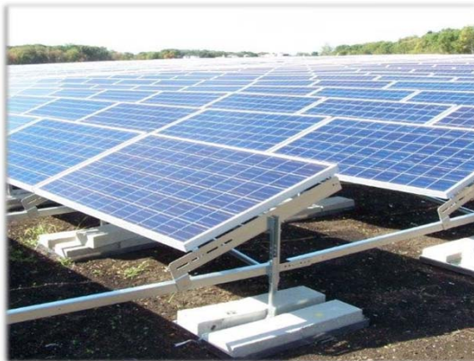
Photo: Solar Energy Panels
