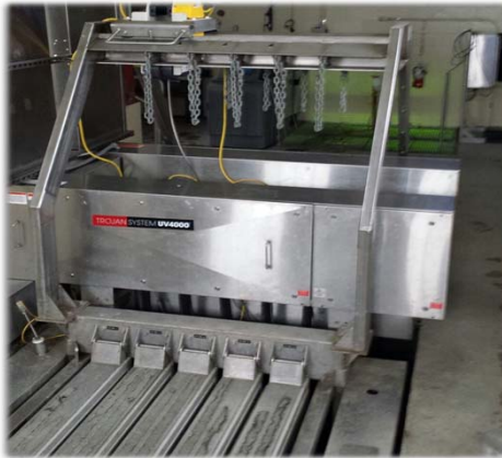
Photo: UV System at BPWWTF
