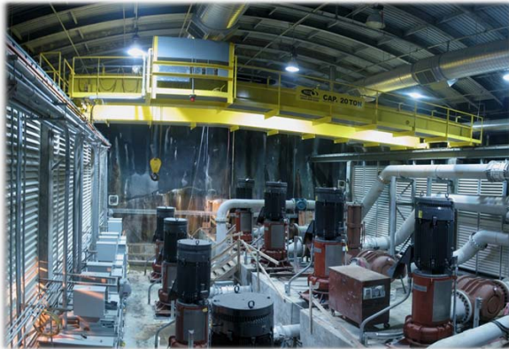
Photo: Tunnel Pump Station Pump Room
