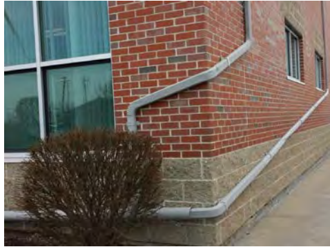
Photo: Downspouts at the NBC COB
