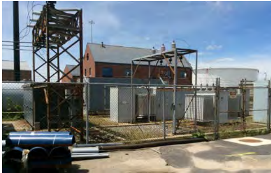
Photo: NBC Facility Electrical Improvements
