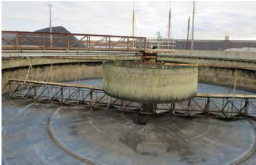
Photo: Final Clarifier at FPWWTF
