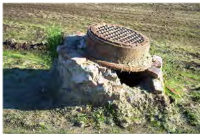
Photo: Inverted manhole cover
