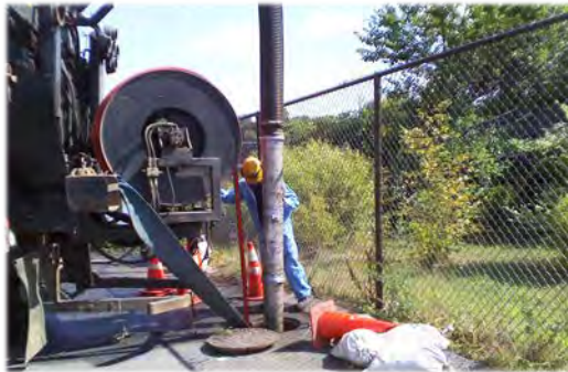
Photo: Interceptor grit removal
