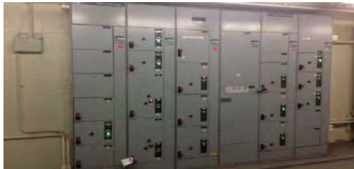
Photo: Field's Point Electrical Panel
