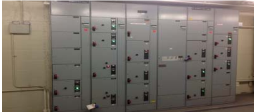
Photo: Field's Point Electrical Panel
