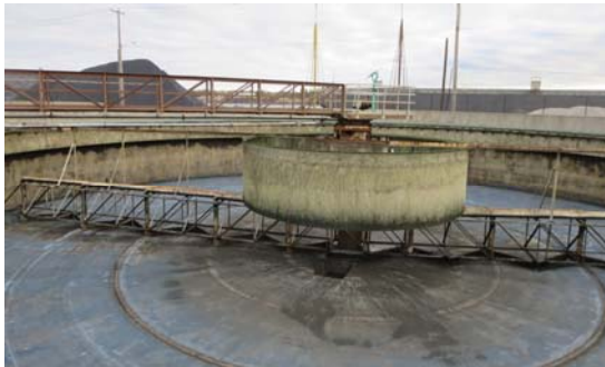
Photo: Final Clarifier at FPWWTF
