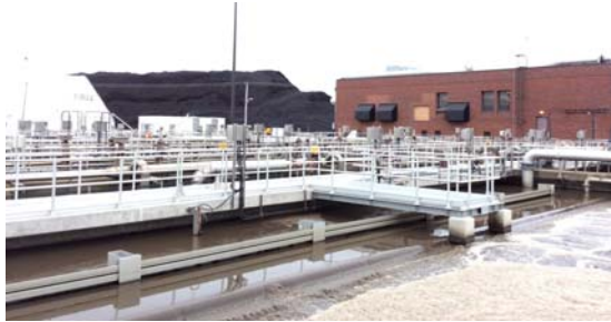
Photo: Aeration tanks at Field's Point
