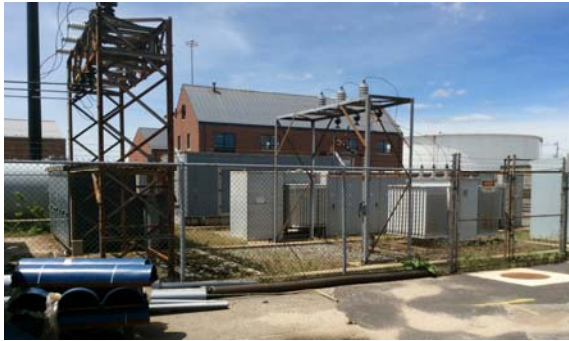
Photo: NBC Facility Electrical Improvements
