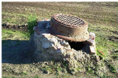
Photo: Inverted manhole cover
