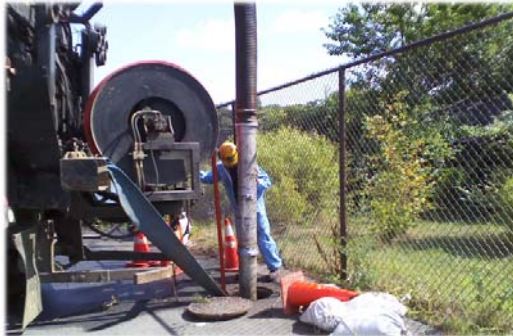
Photo: Interceptor grit removal
