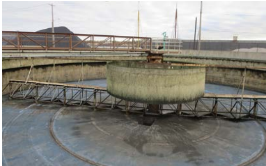
Photo: Final Clarifier at FPWWTF
