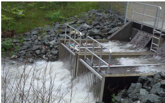
Photo: Floatables Control Facility
