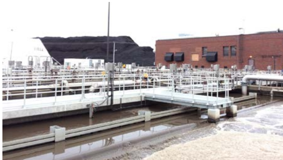
Photo: Aeration tanks at Field's Point
