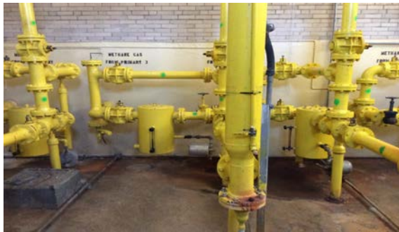
Photo: Existing Digester Methane Piping
