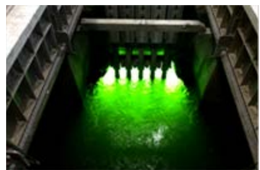
Photo: Ultraviolet Disinfection System
