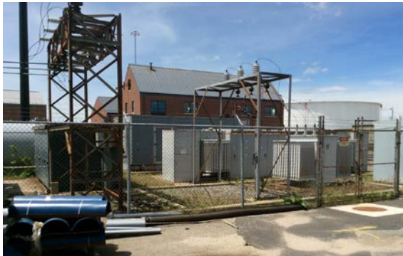
Photo: NBC FPWWTF Electrical Facilities
