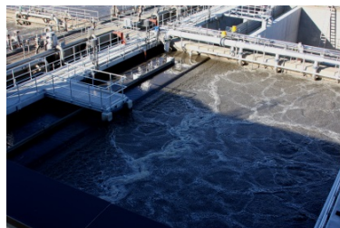
Photo: WWTF Aeration Tank
