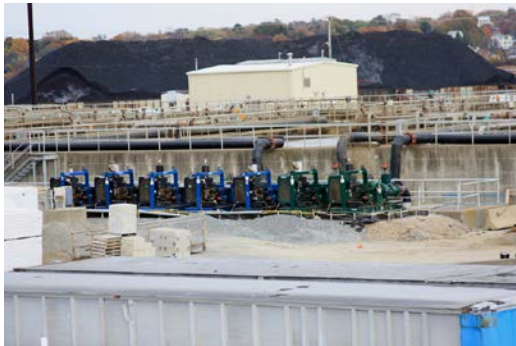
Photo: Aeration Tank Pumps
