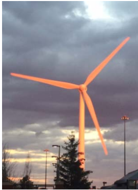
Photo: One of Three Field's Point Wind Turbines
