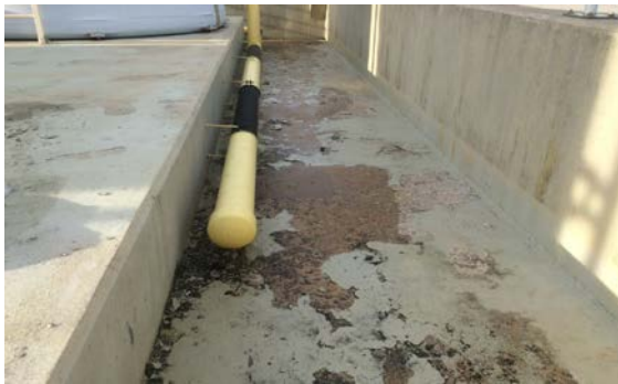
Photo: Hypochlorite Tank Pad
