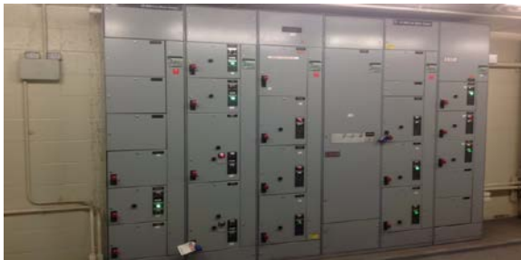
Photo: Field's Point Electrical Panel
