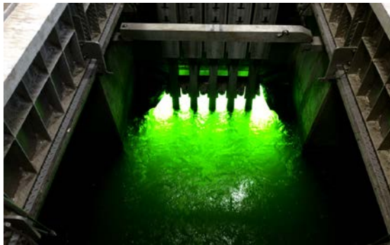
Photo: Ultraviolet Disinfection System
