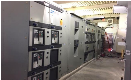
Photo: Motor control center room in blower building
