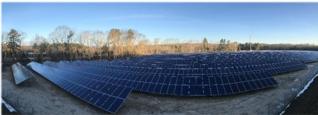
Photo: NBC's Solar Project in Richmond, RI
