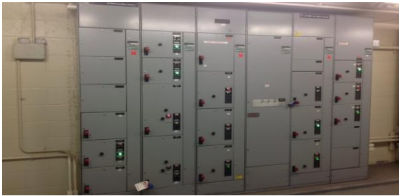
Photo: Field's Point Electrical Panel
