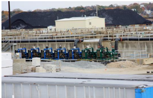
Photo: Aeration Tank Pumps
