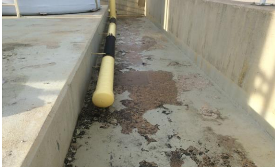
Photo: Hypochlorite Tank Pad
