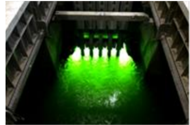
Photo: Ultraviolet Disinfection
