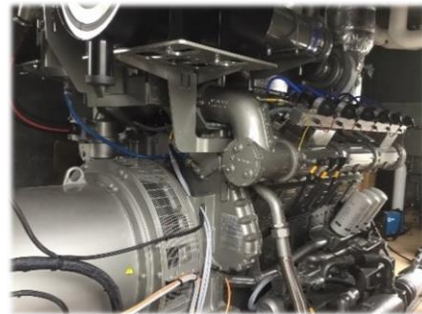
Photo: Bucklin Point Biogas Cogenerator
