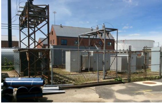
Photo: Field's Point Electrical Switchgear & Transformers
