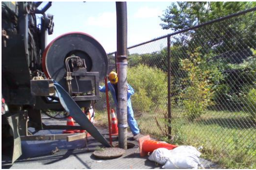
Photo: Interceptor grit removal
