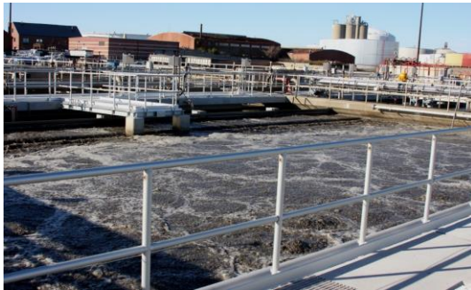
Photo: Aeration Tanks FPWWTF
