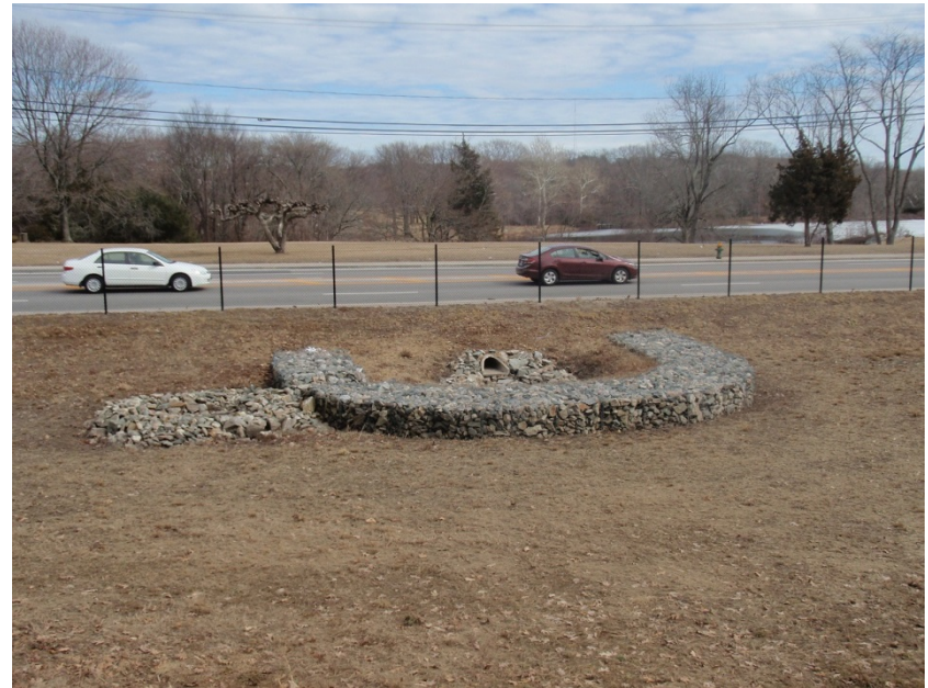
Detention Storage on Atwood Ave Johnston, RI
