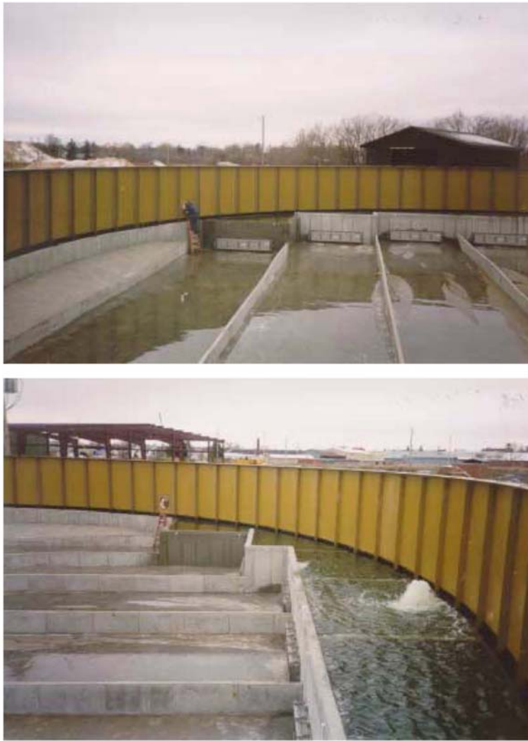
Figure 56 – Circular CSO Storage Tank with Flush Gates
