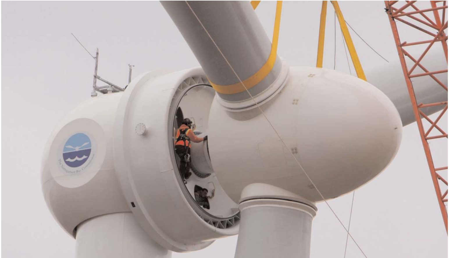
Two hundred and thirty feet up, in the nacell of Tower B, a worker guides the 80,000-pound blade section into place during erection of one of the Narragansett Bay Commission's three 1.5 megawatt wind turbines.
