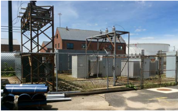
Photo: Field's Point WWTF Electrical Substation #1
