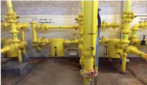
Photo: Existing Digester Methane Piping
