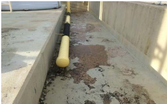
Photo: Hypochlorite Tank Pad
