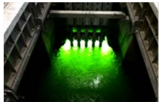
Photo: Ultraviolet Disinfection System
