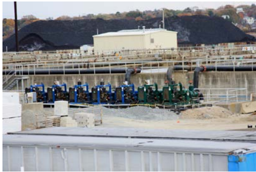
Photo: Aeration Tank Pumps
