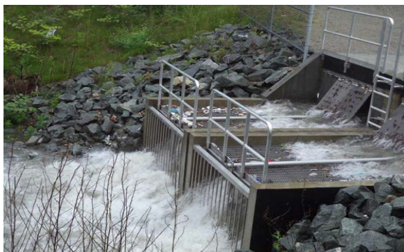
Photo: Floatables Control Facility
