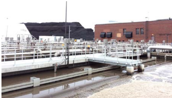
Photo: Aeration tanks at Field's Point
