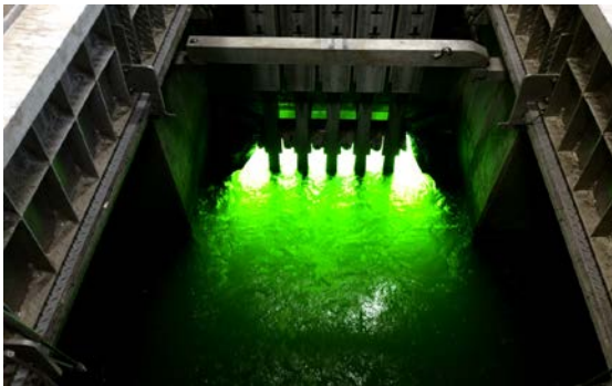
Photo: Ultraviolet Disinfection System
