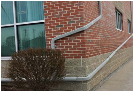
Photo: Downspouts at the NBC COB
