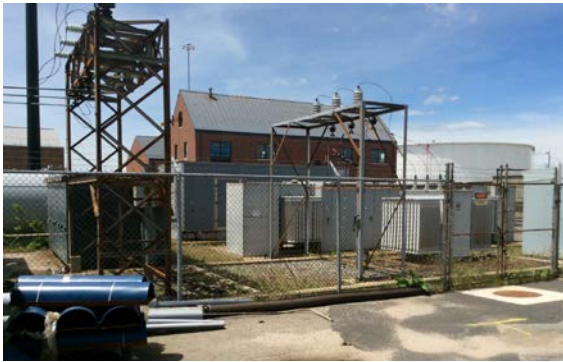
Photo: NBC FPWWTF Electrical Facilities
