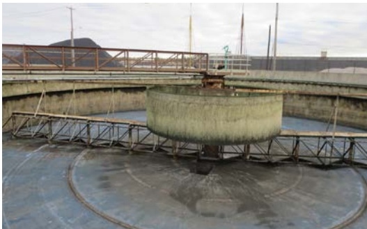
Photo: Final Clarifier at FPWWTF
