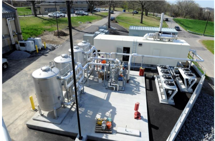
NBC's Biogas CHP installation at Bucklin Point will help NBC attain its goal of utilizing 100% renewable energy for electricity needs.
