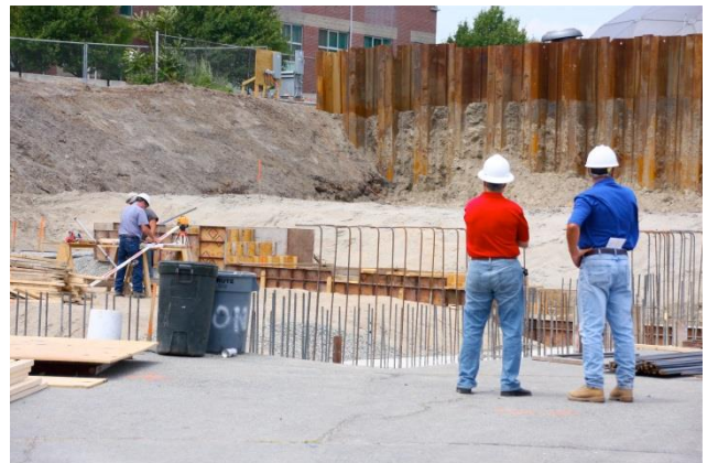
NBC Construction Services staff overseeing the construction of a new building on the NBC Field's Point property.
