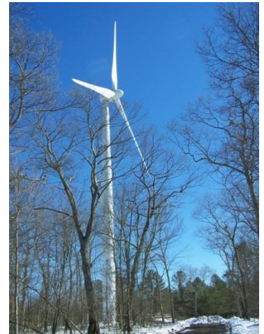
NBC owned wind turbine located in Coventry. The NBC net meters electricity credits from 3 Coventry turbines to help achieve the goal of becoming net-zero.
