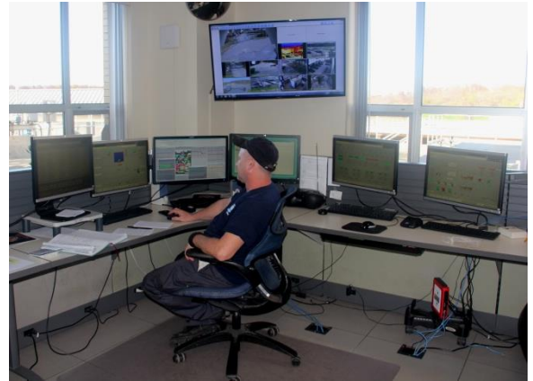
Operations staff monitoring Bucklin Points SCADA systems.
