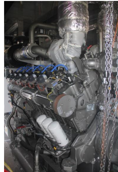
Combined Heat & Power (CHP) generator installed at Bucklin Point to convert biogas to renewable energy.
