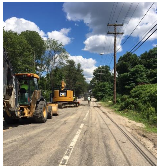
Sewer line installation on Greenville Avenue expanded NBC's service area further into Johnston.
