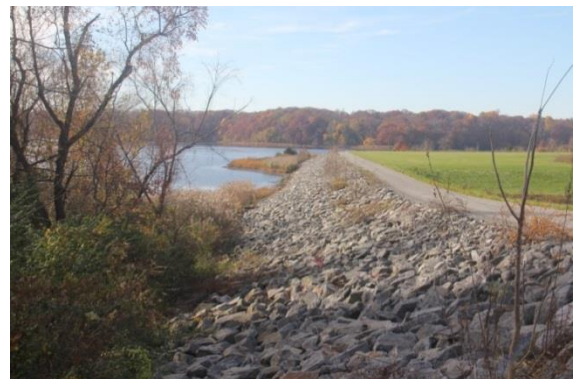
The newly reconstructed berm at Bucklin Point raised the level to better defend against the effects of climate change and sea level rise.
