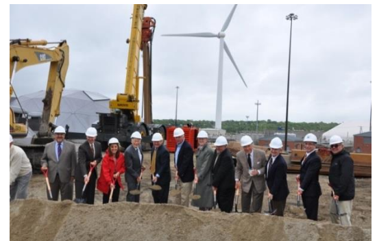
NBC Board of Commissioners breaking ground on NBC's new Water Quality Science Building, a planned capital project.
