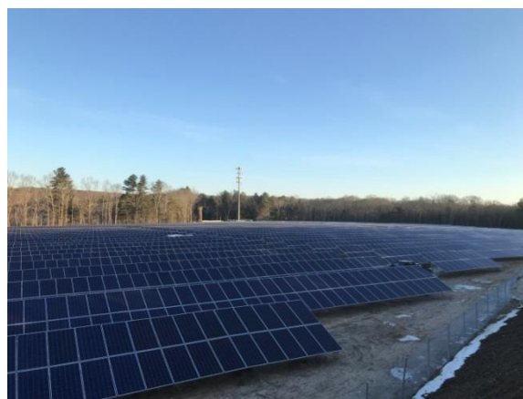
The NBC net meters renewable energy from this solar array facility in Richmond, RI to the electric grid to credit NBC accounts.
