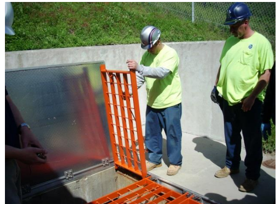
IM staff inspecting NBC facilities to ensure they are functioning properly.
