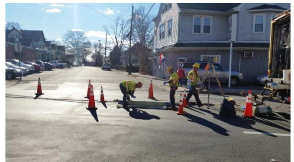
NBC's IM staff inspecting and cleaning lines to increase the capacity of the collection system.
