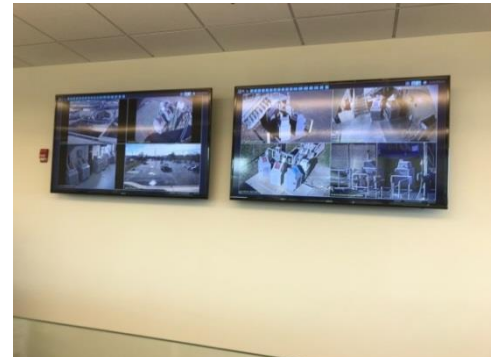
Video monitors in the EMDA office allow oversight of the sampler stations located throughout the treatment plants.
