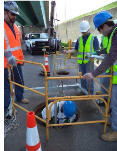
NBC staff regularly receives confined space training to comply with OSHA regulations.
