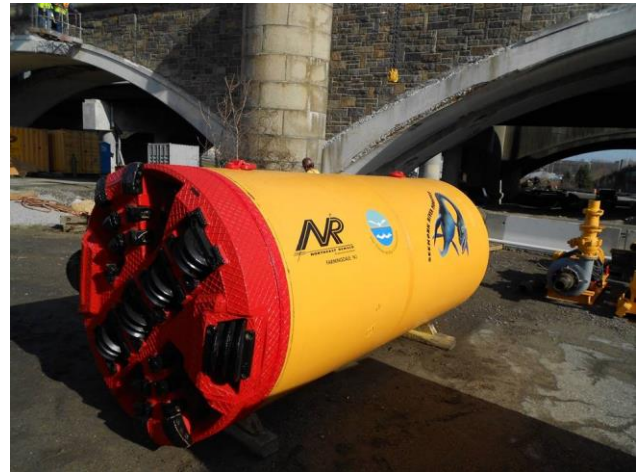
A small tunnel boring machine used in the construction of Phase II of the CSO Abatement Project.
