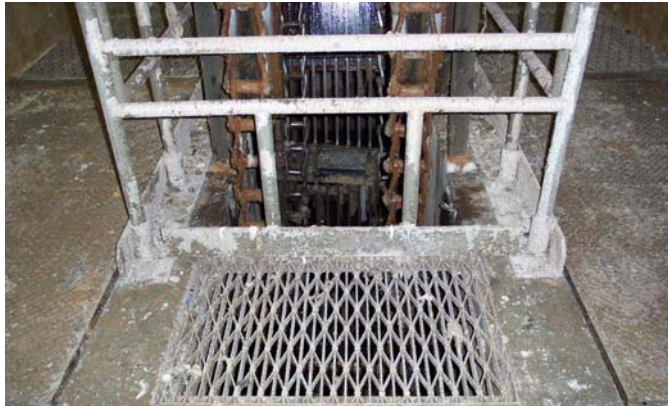
Photo: Bar screen in the Omega rack room
