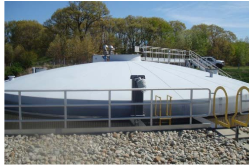
Above: A secondary digester at Bucklin Point
