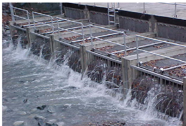
Photo: Floatables Control Facilities at Bucklin Brook
