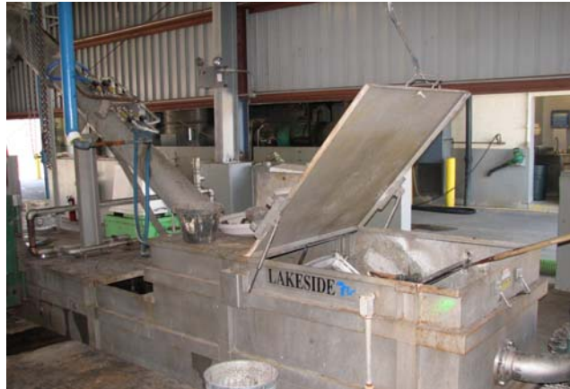
Photo: Lakeside Grit Removal Unit
