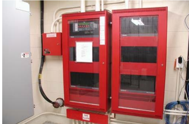
Photo: An existing fire alarm panel from one of NBC's buildings
