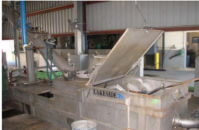
Photo: Lakeside Grit Removal Unit
