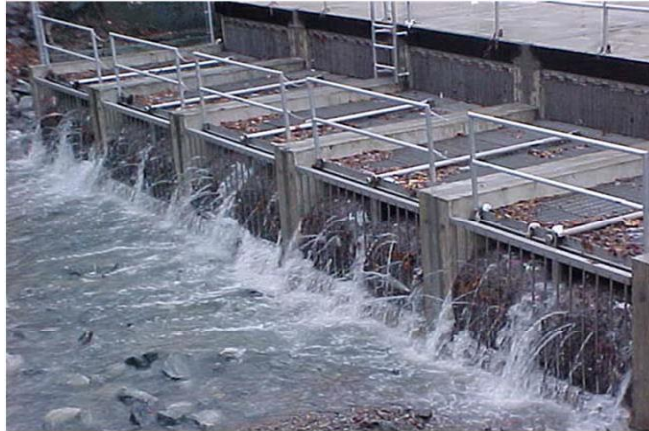
Photo: Floatables Control Facilities at Bucklin Brook
