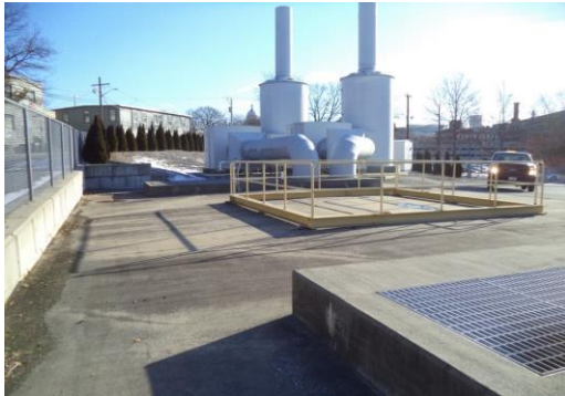
Photo: CSO Tunnel Odor Control Facility
