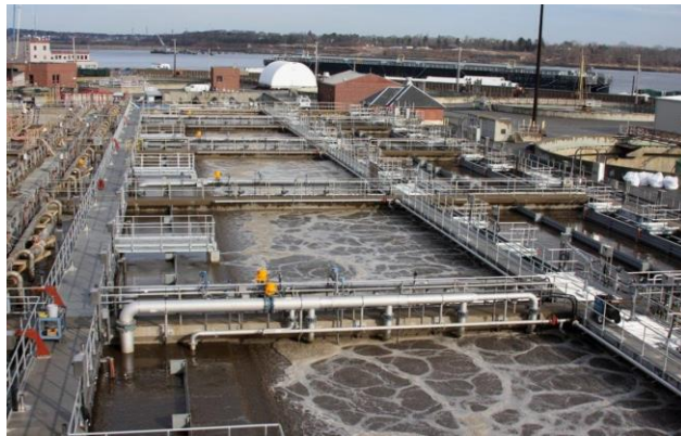
Photo: Aeration Tanks at Field's Point WWTF
