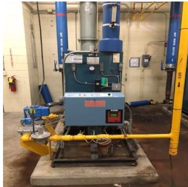
Photo: Screening and Grit Boilers
