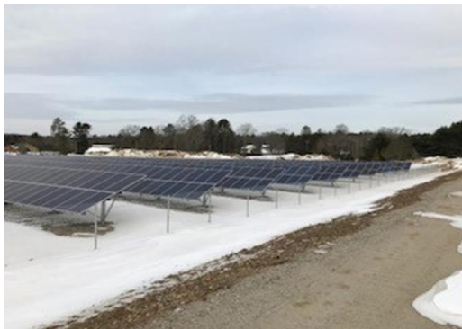
Photo: Solar Panels
