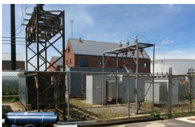
Photo: Field's Point Electrical Facility
