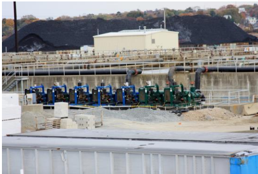
Photo: Aeration Tank Pumps
