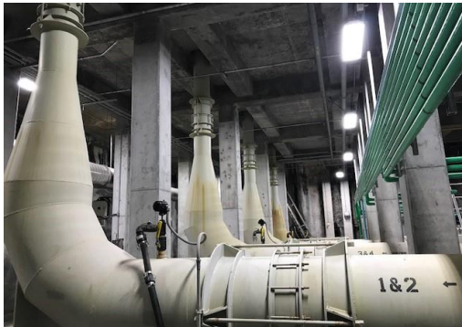
Photo: Inside Ernest St. Tunnel Pump Station
