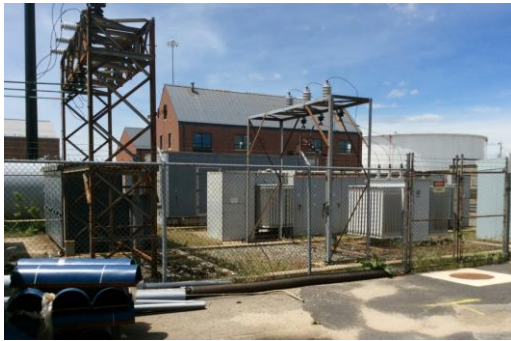
Photo: Field's Point Electrical Facility
