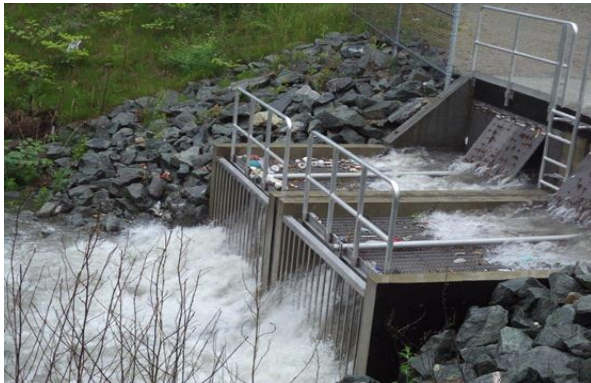
Photo: Floatables Control Facility
