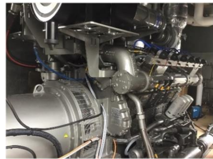
Photo: Bucklin Point Biogas Cogenerator
