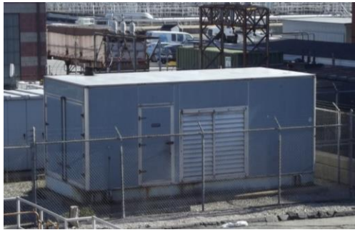
Photo: Field's Point Electrical Facility
