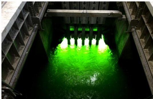
Photo: UV Disinfection System
