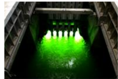
Photo: Ultraviolet Disinfection System at Bucklin Point
