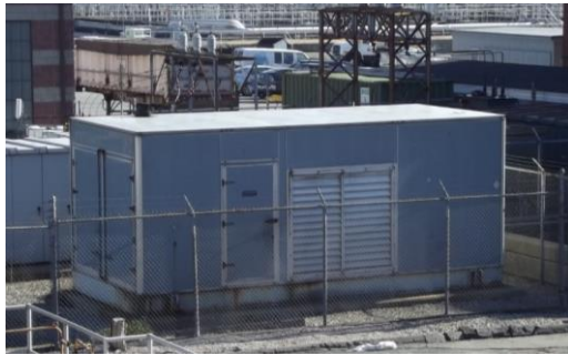
Photo: Field's Point Electrical Facilities
