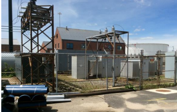
Photo: Field's Point Electrical Switchgear & Transformers
