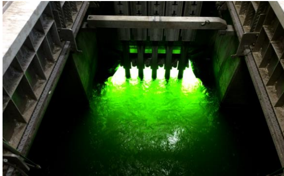
Photo: Ultraviolet Disinfection System
