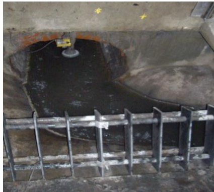
Photo: Flow Meter Installed
