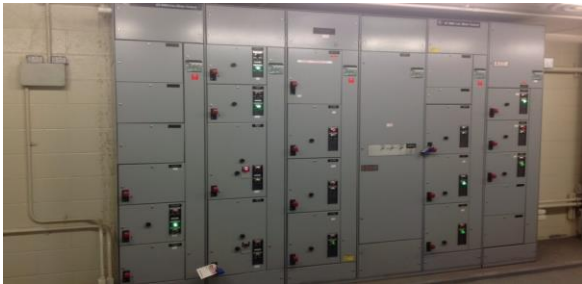
Photo: Field's Point Electrical Panel
