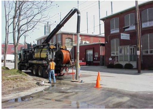
Photo: Interceptor Grit Removal
