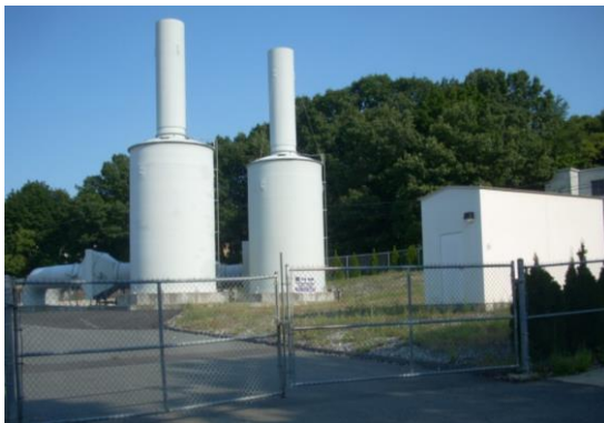
Photo: CSO Tunnel Odor Control Facility
