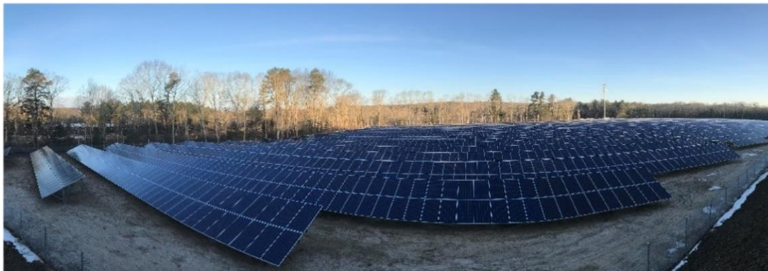
Photo: NBC's Solar Facilities in North Kingstown, RI
