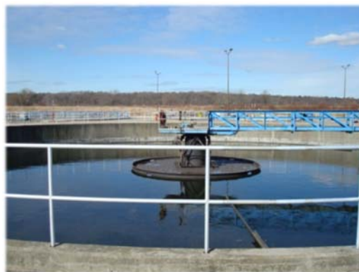
Photo: Final clarifier tank at Bucklin Point
