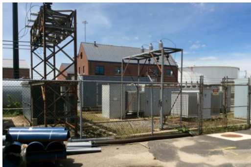
Photo: Field's Point Electrical Facility
