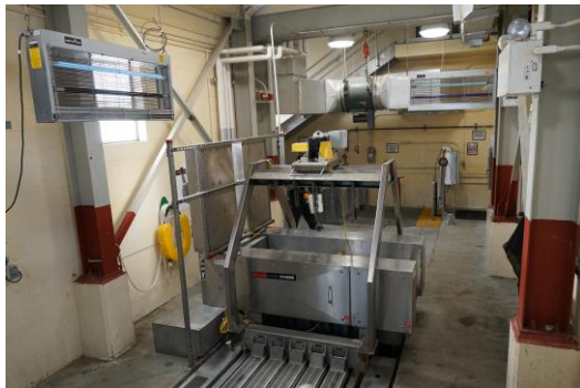
Photo: Bucklin Point UV Disinfection System
