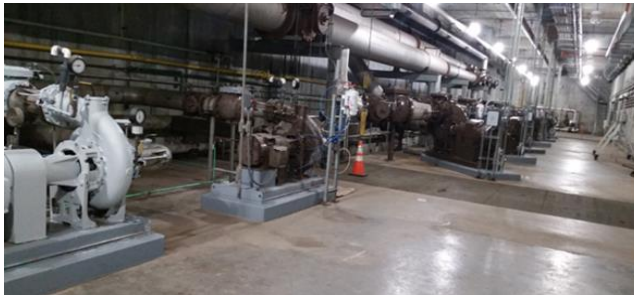
Photo: RAS Pumps
