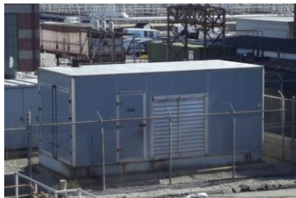
Photo: Field's Point Electrical Facility
