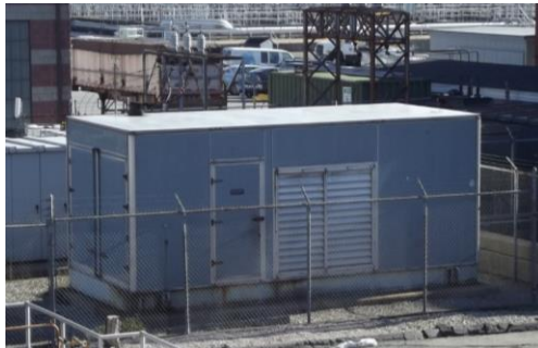
Photo: Field's Point Electrical Facility
