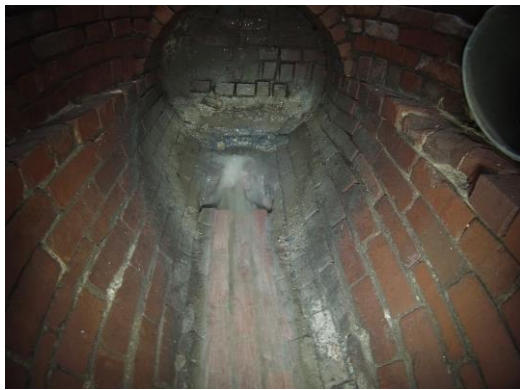
Photo: OF 056 Regulator on Vandewater Street
