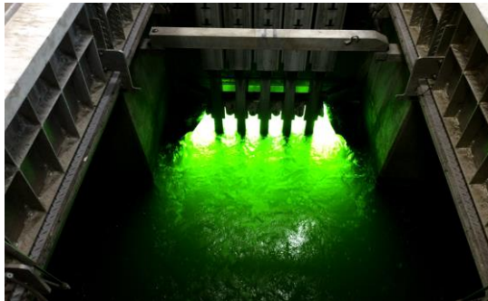
Photo: UV Disinfection System
