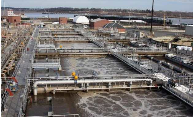
Photo: Aeration Tanks at Field's Point WWTF
