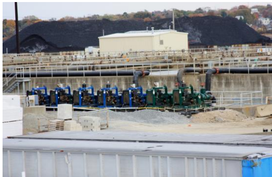
Photo: Aeration Tank Pumps
