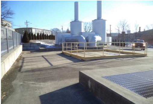
Photo: CSO Tunnel Odor Control Facility
