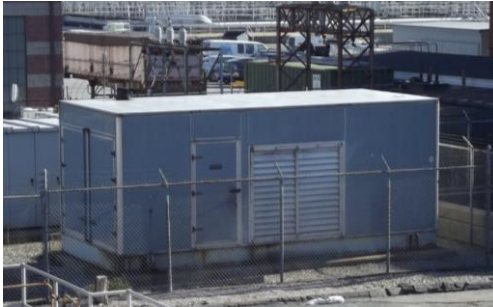
Photo: Field's Point Electrical Facility
