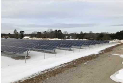
Photo: Solar Panels
