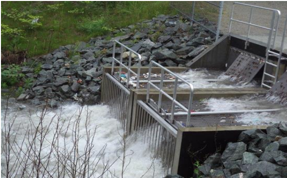
Photo: Floatables Control Facility
