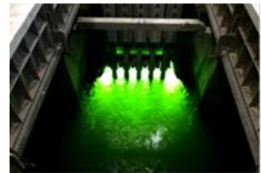
Photo: Ultraviolet Disinfection System at Bucklin Point
