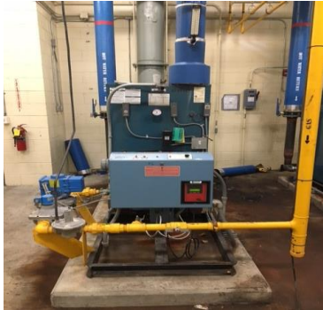
Photo: Screening and Grit Boilers
