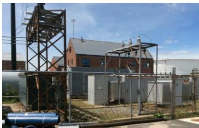
Photo: Field's Point Electrical Facility
