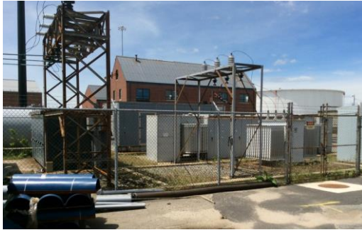
Photo: Field's Point Electrical Facility
