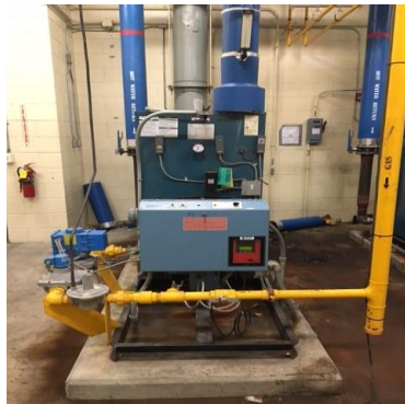
Photo: Screening and Grit Boilers
