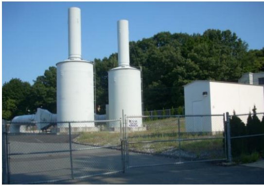
Photo: CSO Tunnel Odor Control Facility
