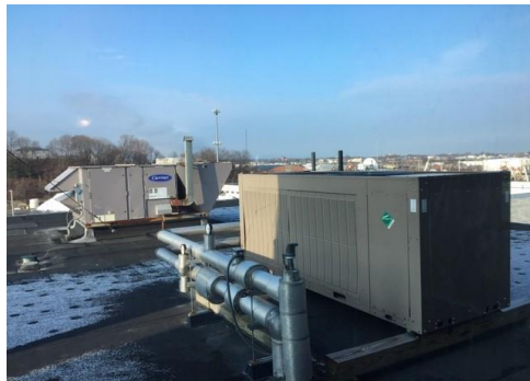
Photo: HVAC Units at COB
