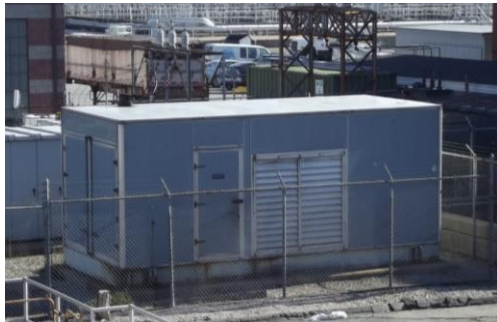
Photo: Field's Point Electrical Facility
