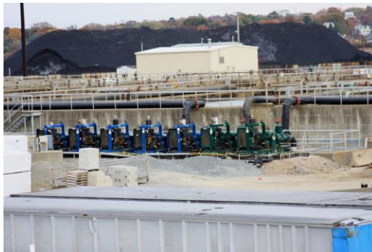
Photo: Aeration Tank Pumps
