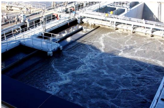
Photo: Aeration Tanks at Field's Point WWTF
