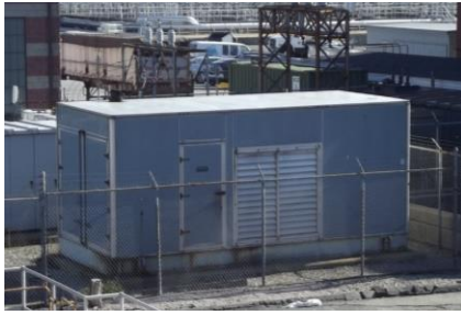
Photo: Field's Point Electrical Facility
