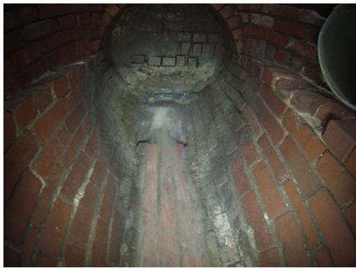
Photo: OF 056 Regulator on Vandewater Street
