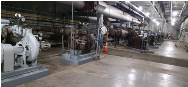
Photo: RAS Pumps
