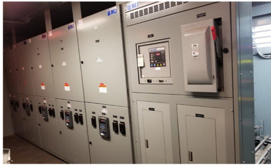
Photo: Field's Point Electrical Facility
