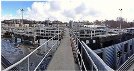
Photo: Aeration Tanks at the Fields Point Wastewater Treatment Facility
