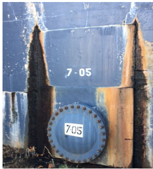
Photo: Secondary Digester
