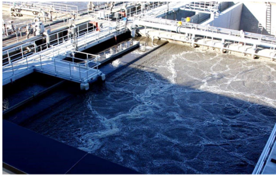
Photo: Aeration Tanks at Field's Point WWTFF
