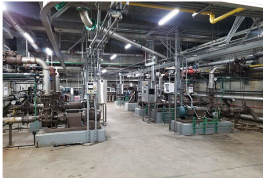
Photo: Primary Pump Station
