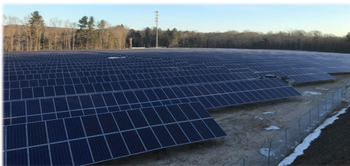
Photo: NBC's Solar PPA Facilities in North Kingstown, RI
