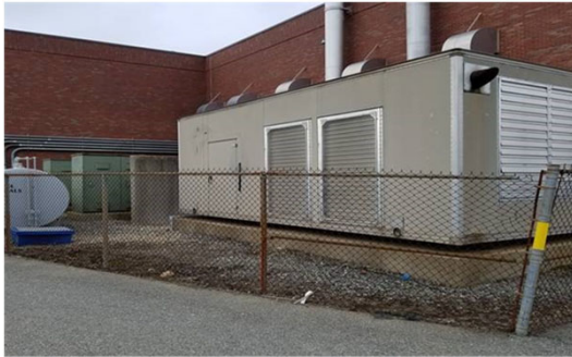
Photo: Field's Point Screw & Blower Generator
