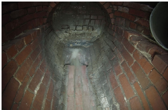
Photo: OF 056 Regulator on Vandewater Street
