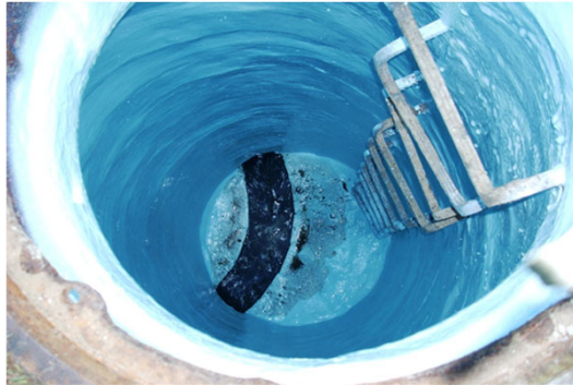
Photo: Flow Monitor
