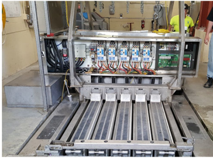
Photo: Bucklin Point UV Disinfection System
