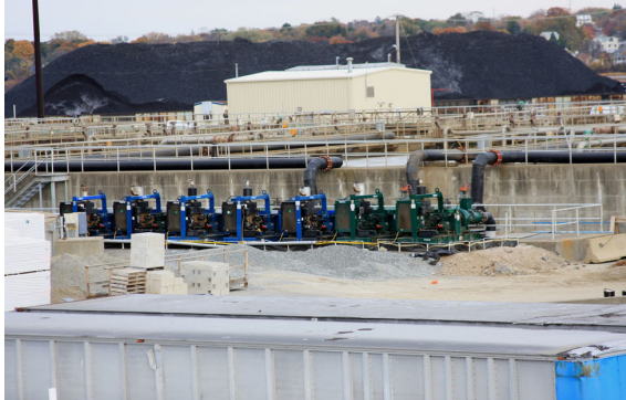
Photo: Aeration Tank Pumps
