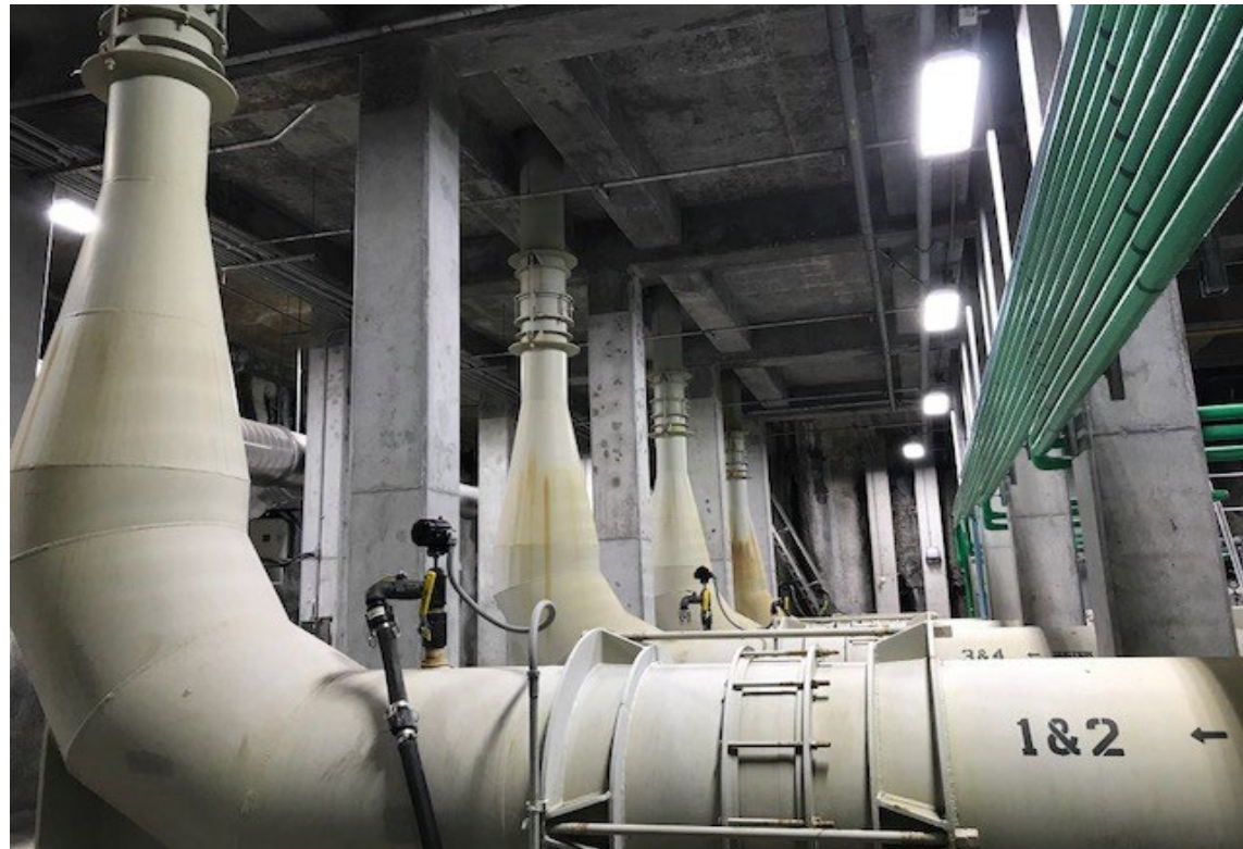
Photo: Ernest Street Tunnel Pump Station
