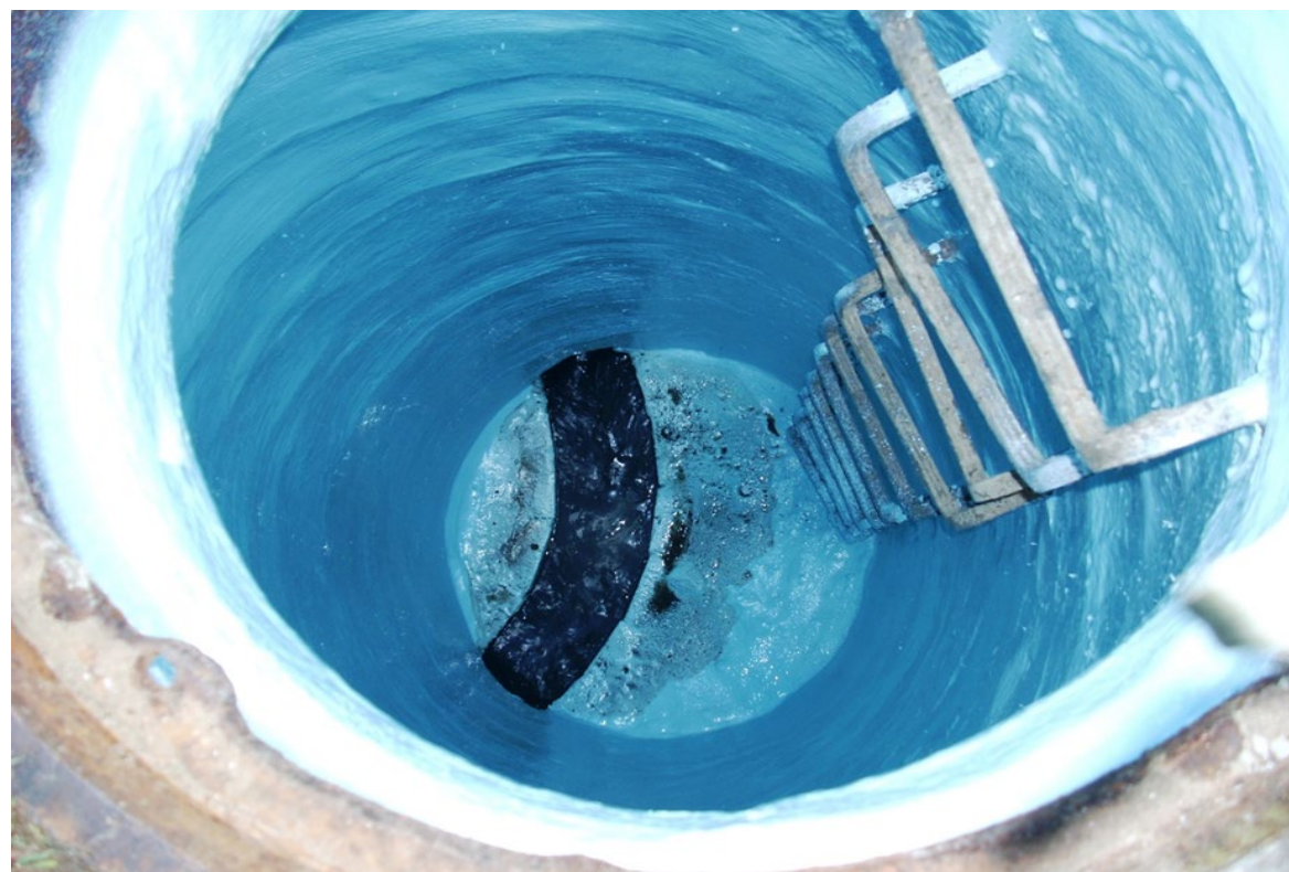
Photo: Flow Monitor
