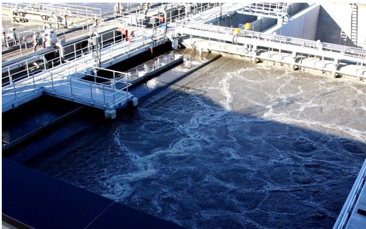
Photo: Aeration Tanks at Field's Point WWTF
