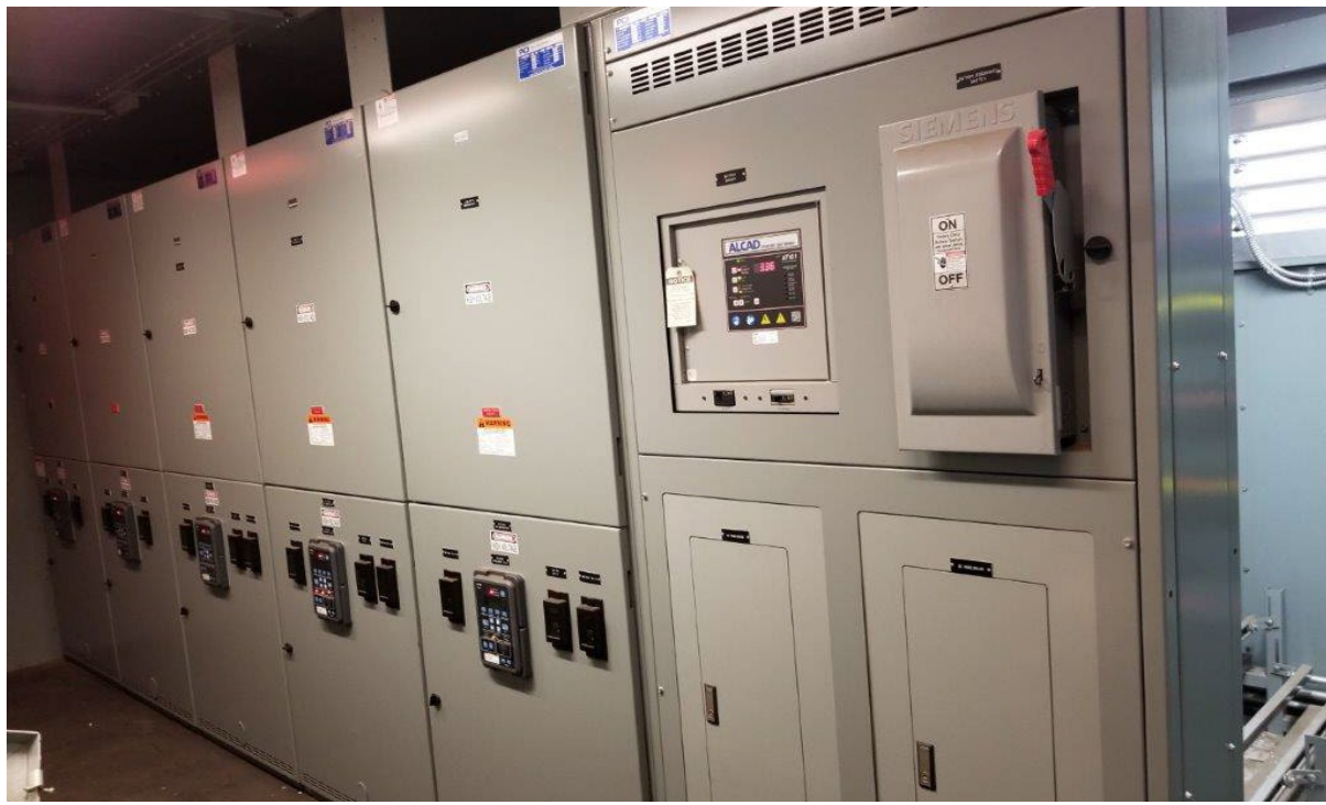
Photo: Field's Point Electrical Facility
