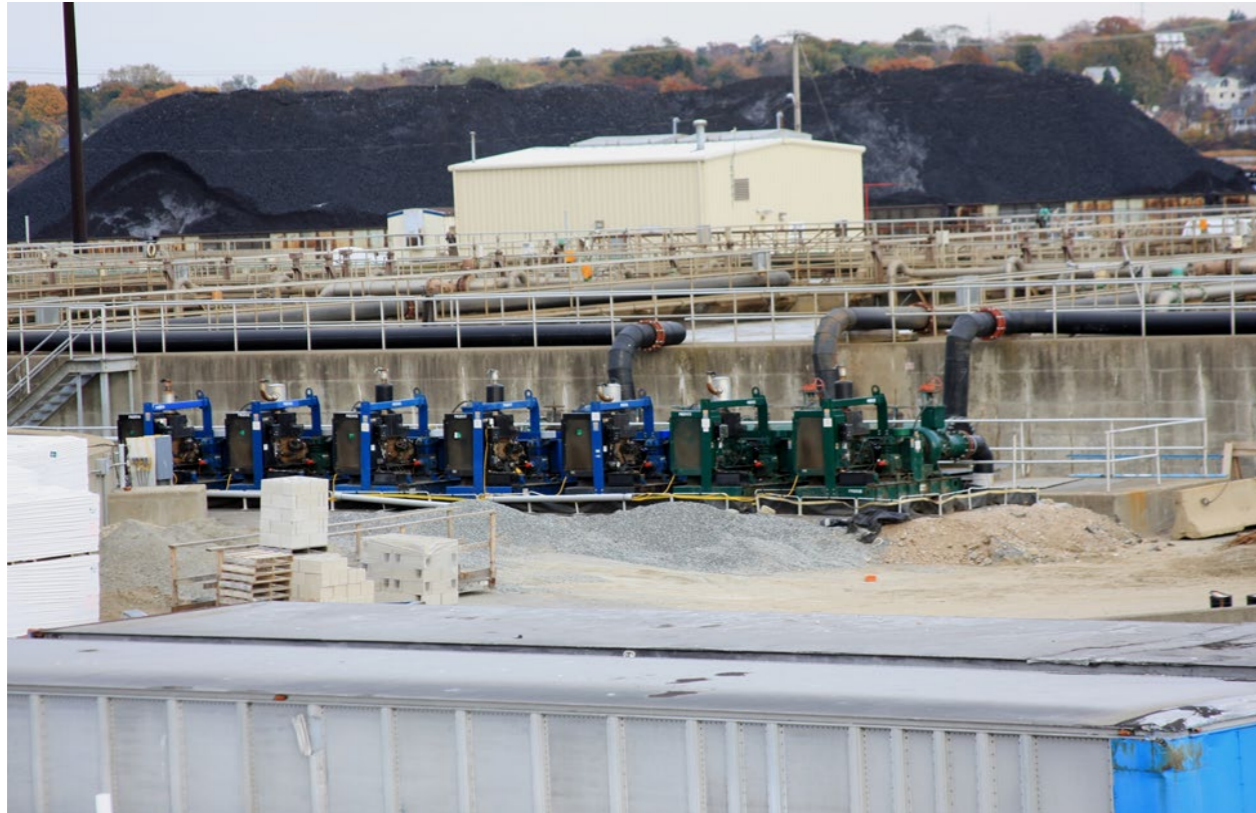
Photo: Aeration Tank Pumps
