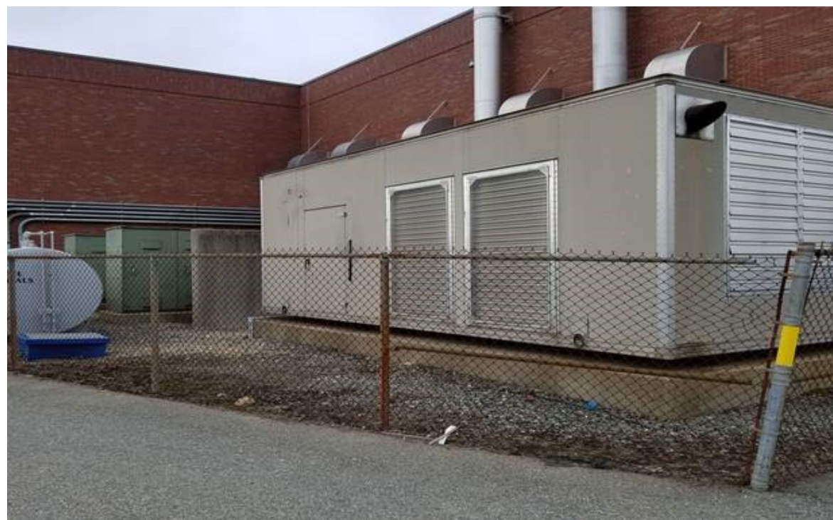
Photo: Field's Point Screw & Blower Generator
