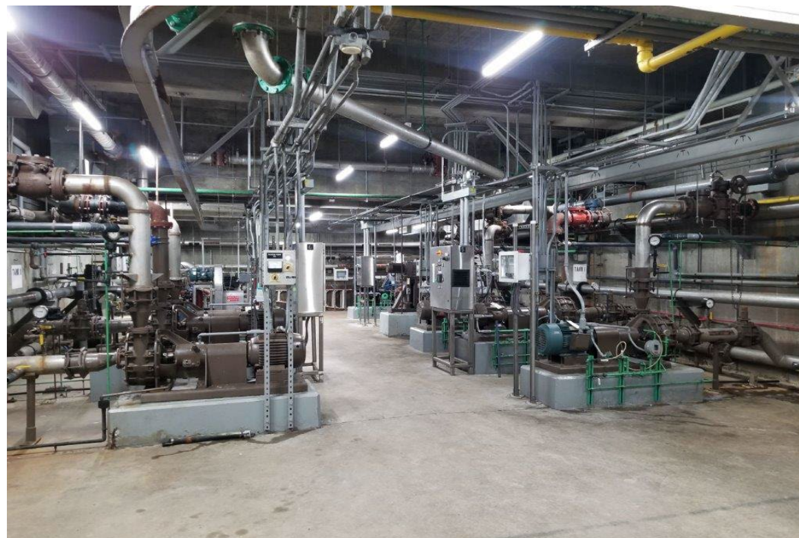
Photo: Primary Pump Station
