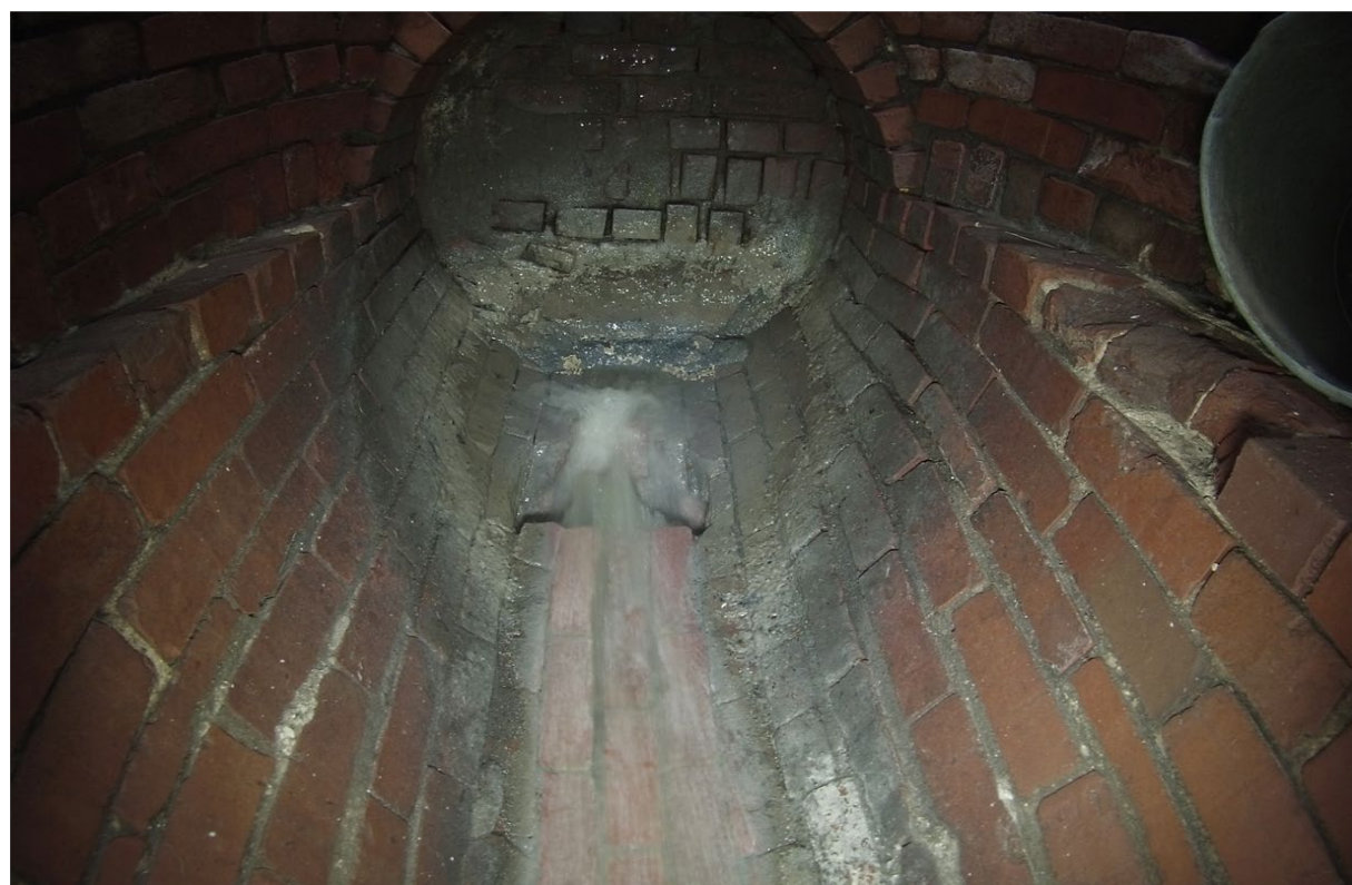
Photo: OF 056 Regulator on Vandewater Street
