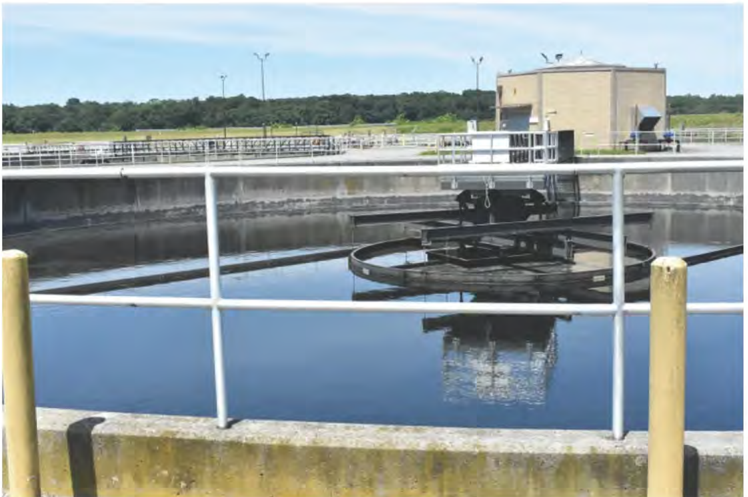
The NBC's wastewater treatment plant at Bucklin Point
