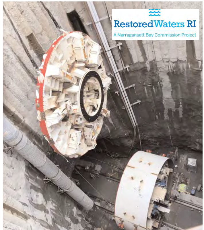
TBM cutterhead being lowered into the main drop shaft at 804 School Street, Pawtucket. Photo courtesy of Stantec.
